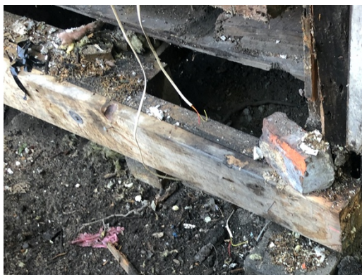
P7: Floor Structure Deterioration
