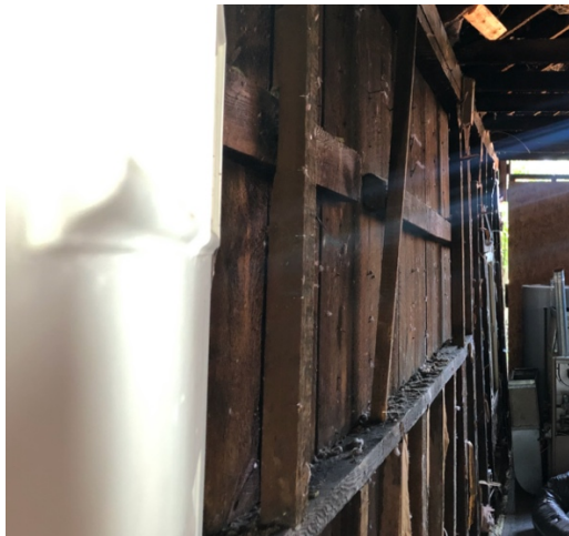
P2: Bearing Wall Leaning
