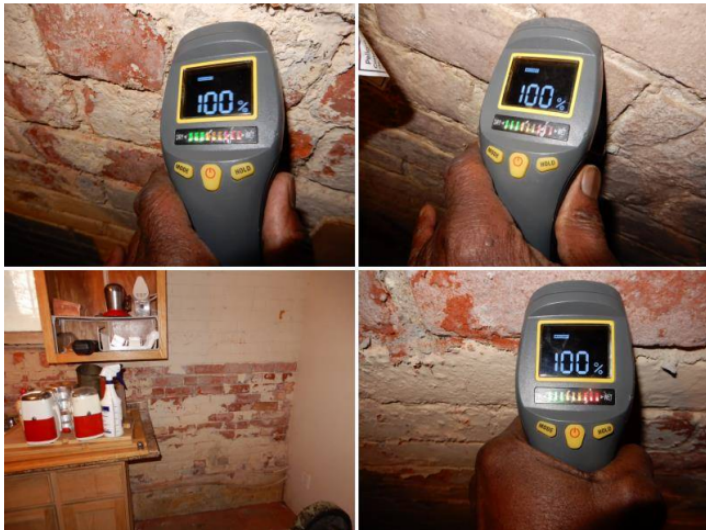
Measurements of water in bricks during home inspection prior to purchase.
