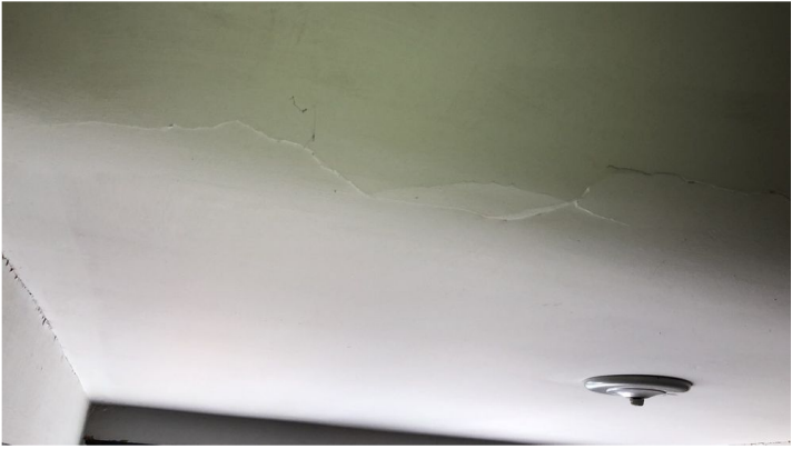
Project: Fay, Evan Date: June 20th, 2020, 11:14 a.m. Creator: Mason Mahaffey
