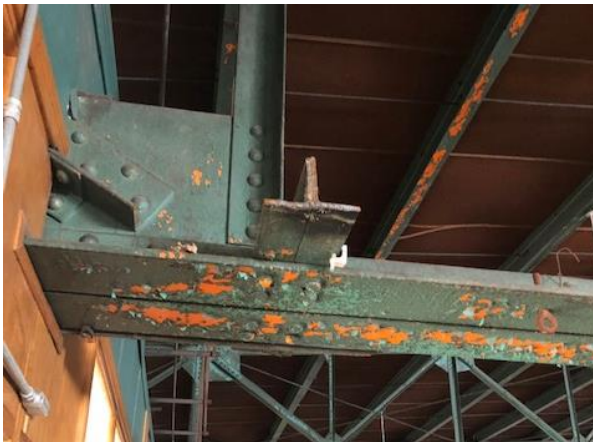
P-12 Removed bottom chord bridging
