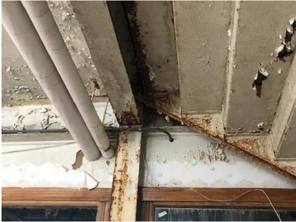
P-7 Corroded stair stringer and connection
