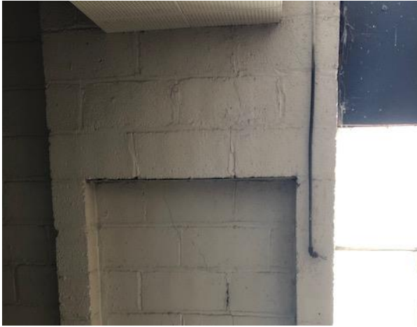
P-16 Hairline cracking at truss bearing pocket
