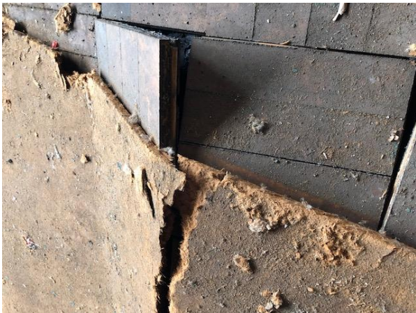
P-18 Fallen section of roof decking
