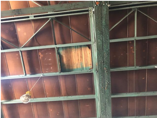
P-17 Deteriorated roof decking
