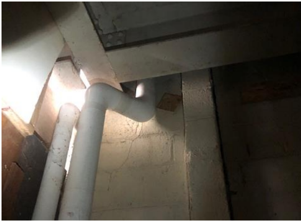
P-8 Masonry wall crack at bearing pocket
