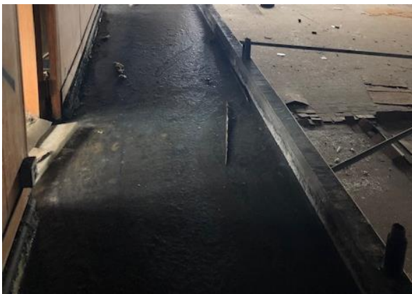
P-9 Missing guardrail
