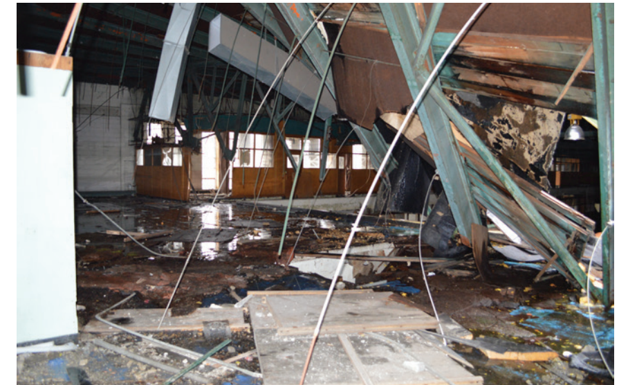
Roof collapse in the Main Drill Hill (Jefferson Avenue Block); scrappers removed bottom chord of roof truss
