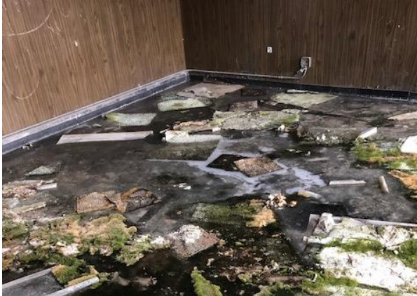
P-4 Mezzanine structural slab water ponding
