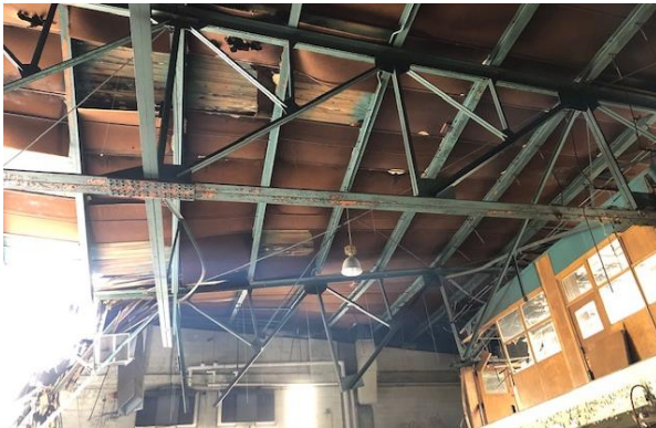
P-11 Removed truss bottom chord (1 st truss)
