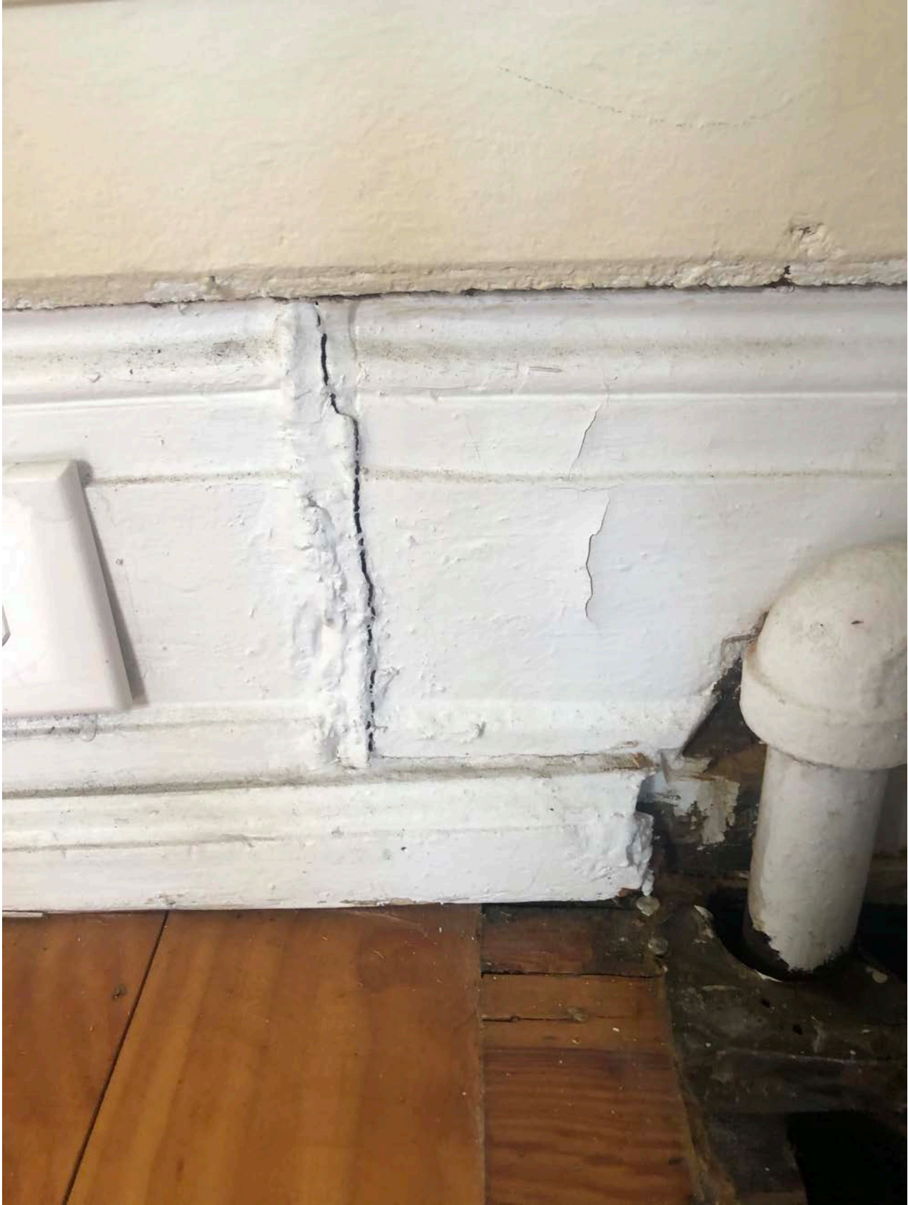
INTERIOR 2ND FLOOR DAMAGE
