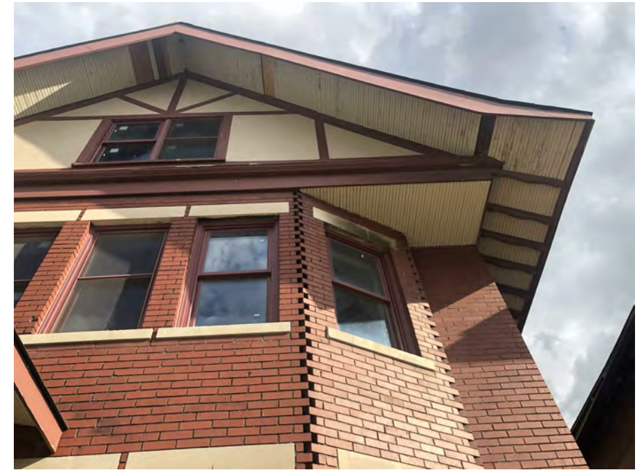
3. EXISTING CONDITIONS AT GABLE
