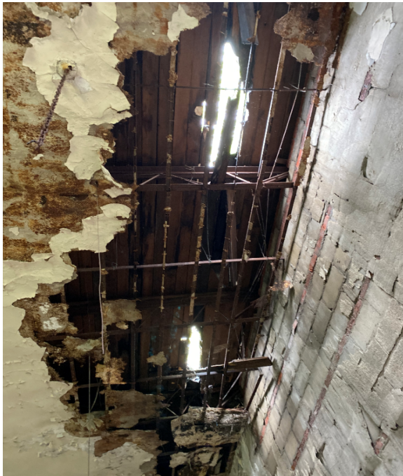
Roof damage, as viewed from inside the building
