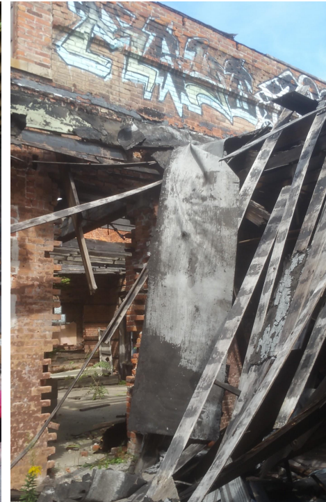
FROM 1-STORY INTO CARRIAGE (ROOF COLLAPSED)
