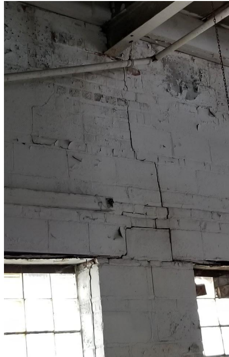
INTERIOR LOOKING EAST (COMPROMISED STRUCTURE)
