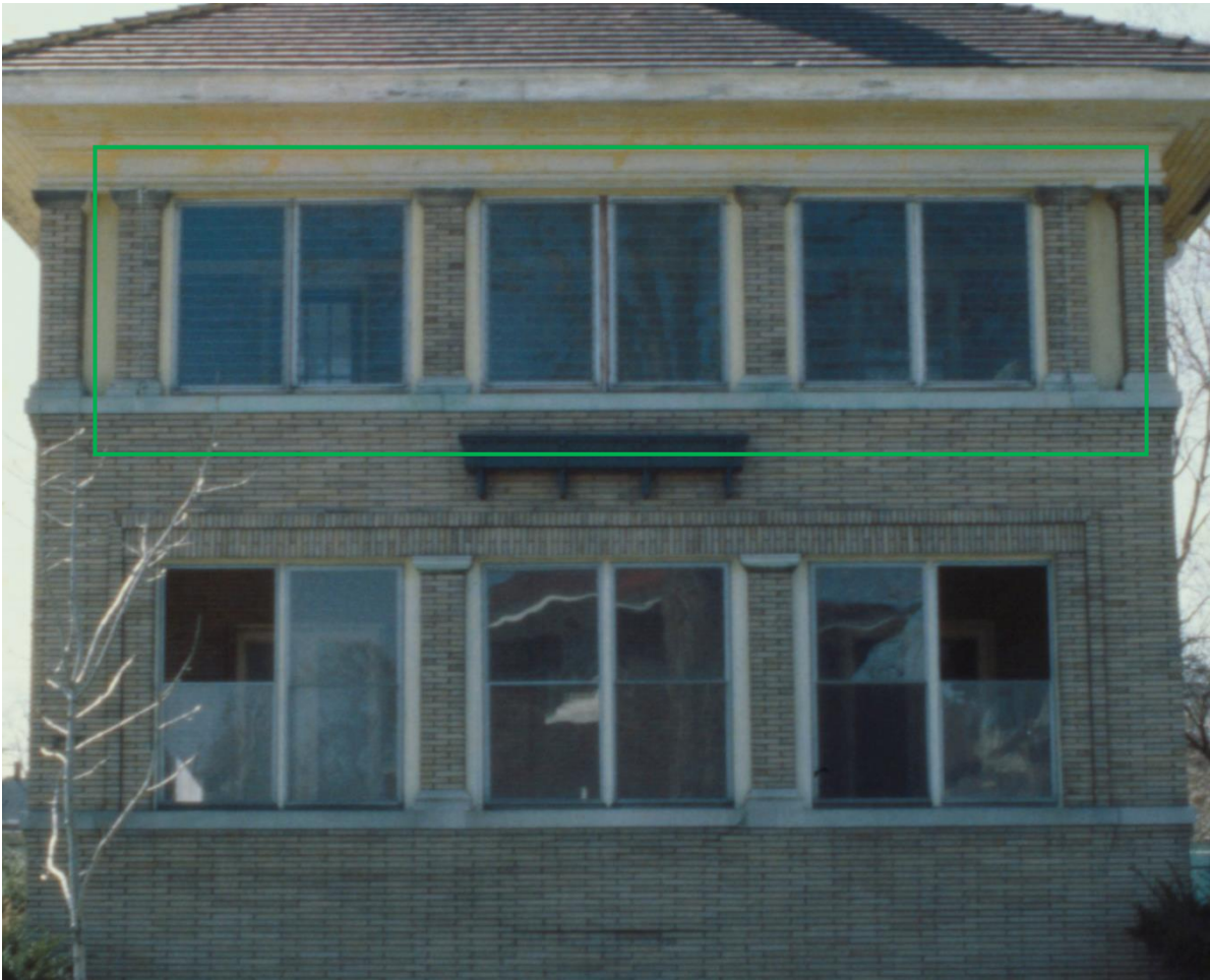
801 Edison, photo taken in 1980. See the side porch wing. The windows at the porch outlined in green are jalousie windows. All other windows at the porch appear to be 1/1 storm windows
