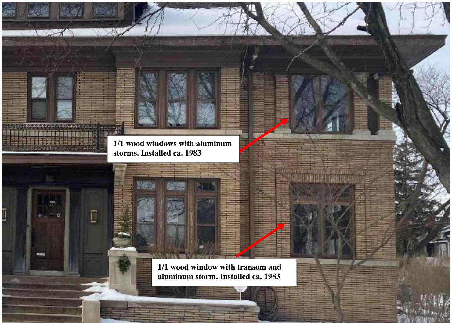
East/front façade, showing windows at porch which are proposed for replacement. Staff photo taken on 2/25/2025
