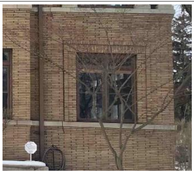
Above referenced porch window opening at front façade, first story, current condition. This window was installed ca. 1983
