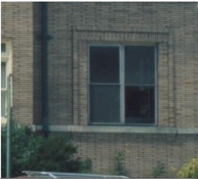
Above referenced porch window opening at front façade, first story, condition in 1974, prior to ca. 1983 replacement
