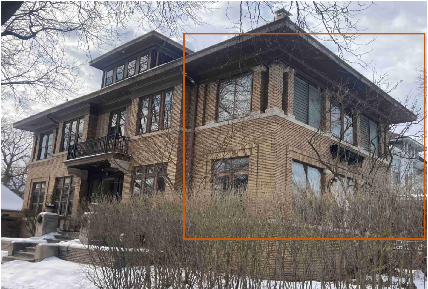
801 Edison, current conditions. Photo by HDC staff, 2/25/2025. North side porch outlined in orange
