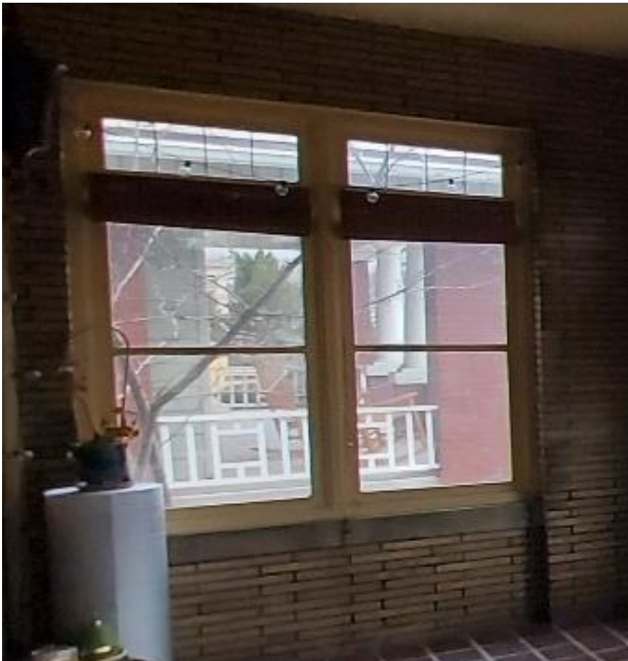
Window type that is present at the porch, front façade, first story. This window was installed ca. 1983. The window type is a wood 1/1 unit with what appears to be a fixed transom with metal caming
