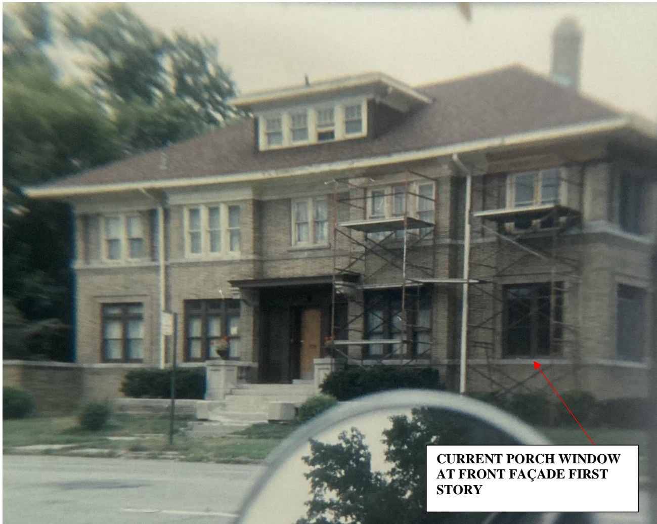
Ca. 1983 photo. Note that the owner was in the process of replacing the side porch windows per the above note. See the below photos to note the window conditions in 1974 and 2025.
