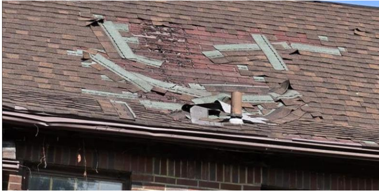
Area of prior roof deterioration. Image from August 22, 2024, application documents for roof repairs.
