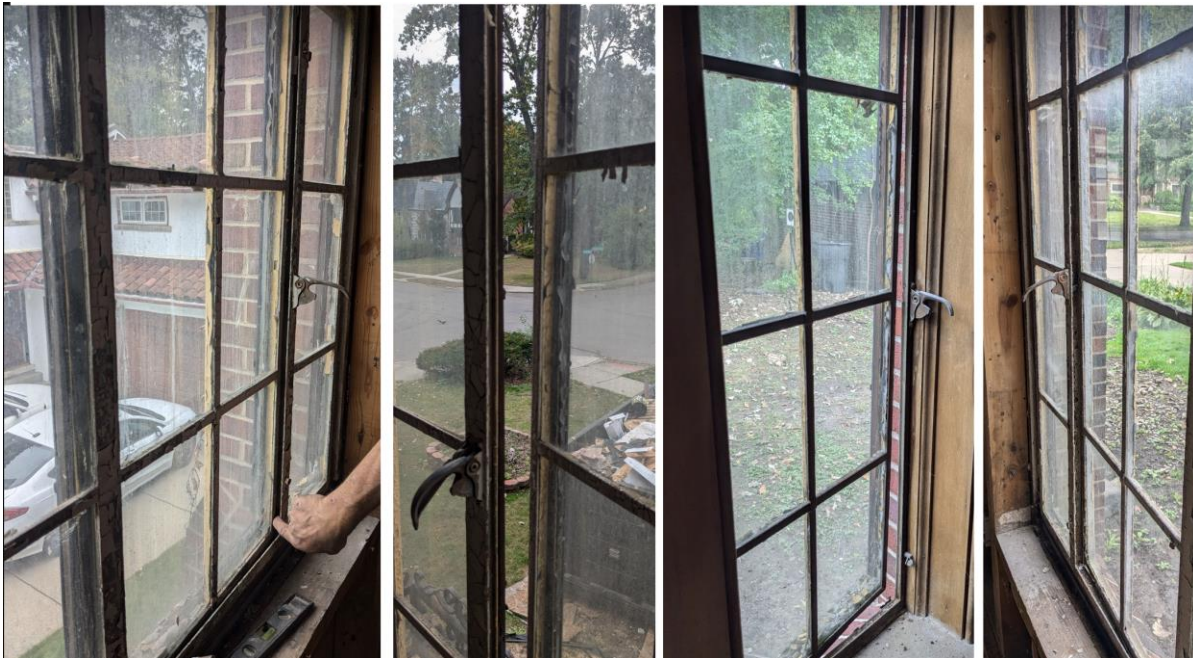
October 2024 staff photos showing warped casements.
