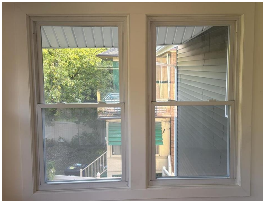
Image, from application documents, showing proposed (already installed) vinyl windows, vinyl siding, vinyl soffit panels, and vinyl gutters and downspouts.
