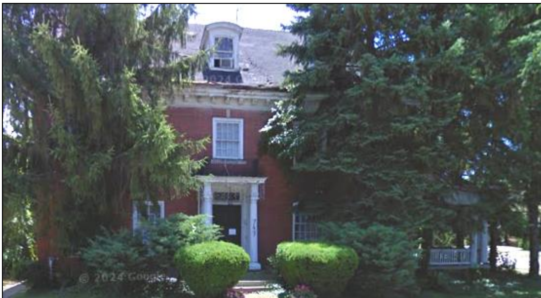
This 2009 Google street view image shows the evergreen trees dwarfing the house. Their proximity to the house coupled with deferred maintenance, exacerbated deterioration to some portions of the façade's eaves, soffits and brackets.
