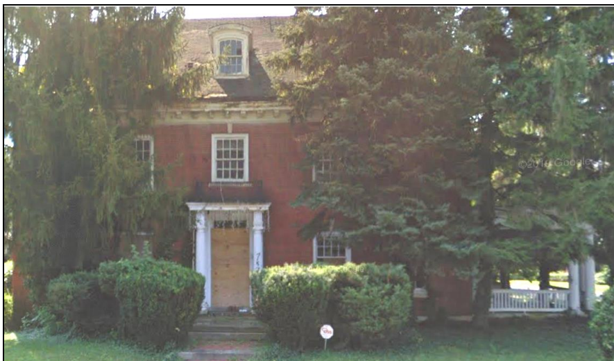
The last documentation of the intact portico is this 2013 Google street view.
