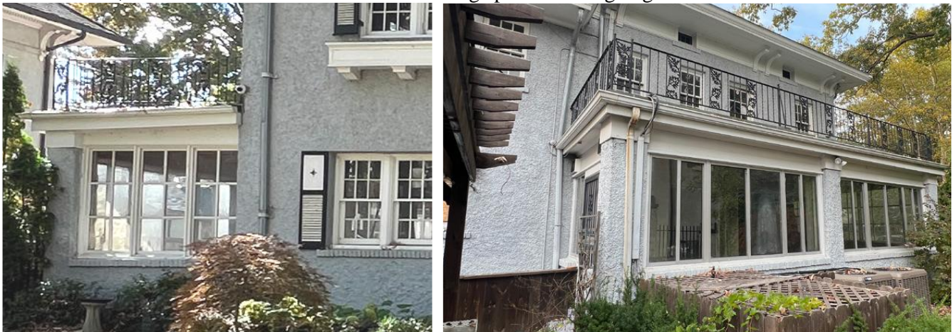
Windows to be retained on the three walls of the south wing. Applicant photos.
