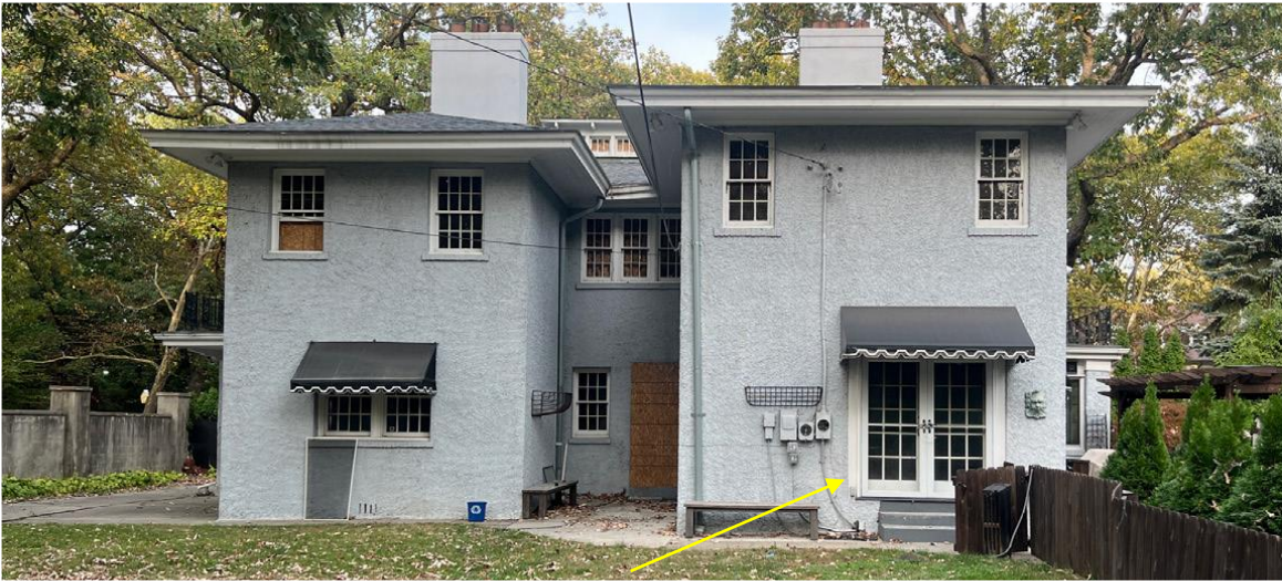
Rear wall of the house. Applicant photo. The French door is proposed for replacement.
