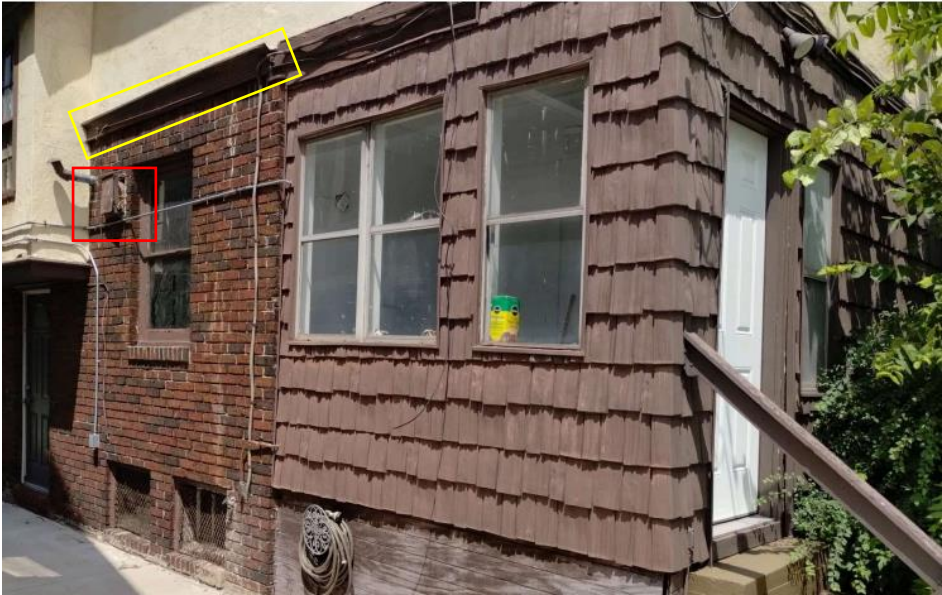
Area of trim proposed for in kind replacement (outlined in yellow) and vent proposed for removal (outlined in red). Photo by applicant
