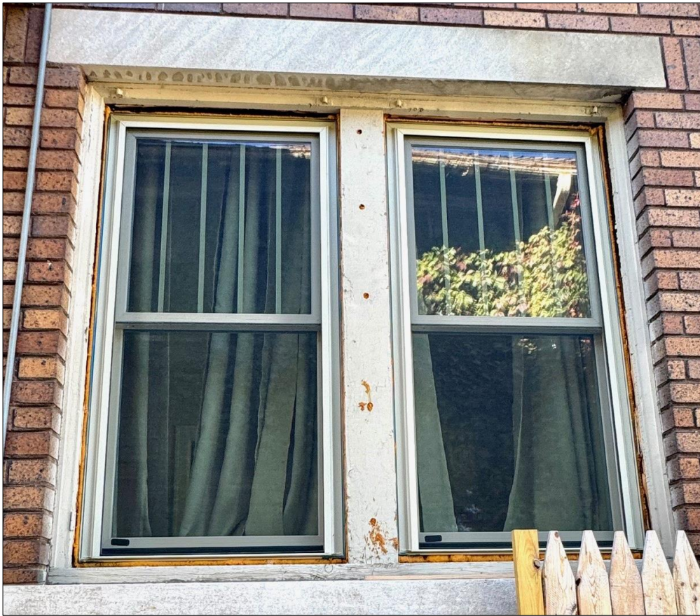
This two-unit window opening is located on the east wall at the rear of the house. The replacement windows are in place and the spray foam applied, but the wood brickmould, central mullion and sill remain exposed.
