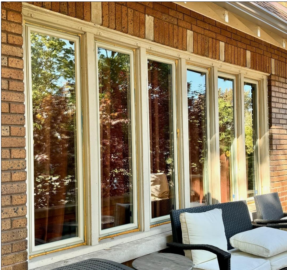
Façade window opening, first floor. These vinyl units replaced non-original, non-approved windows that were installed in 2013 and replaced the original leaded glass casement units. Staff photo, October 9, 2024.
