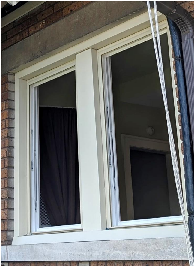
This photo shows two openings that have the vinyl frames in place, but not the sash. The wood brickmould, central mullion and sill has been covered with aluminum coilstock.
