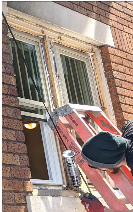
This photo shows the vinyl frames and sash in place, and foam is being added in open areas prior to the wood brickmould, central mullion and sill being covered with aluminum coilstock.
