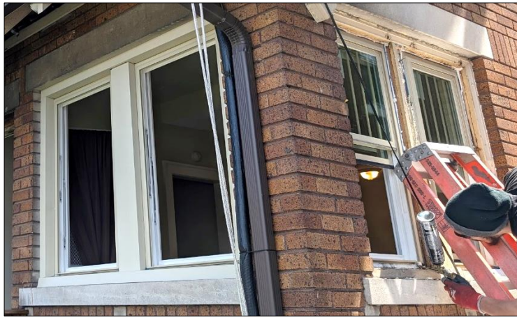
HDC staff photos of in-progress replacement window installation, April 2024. These windows are at the rear northwest corner of the house.
