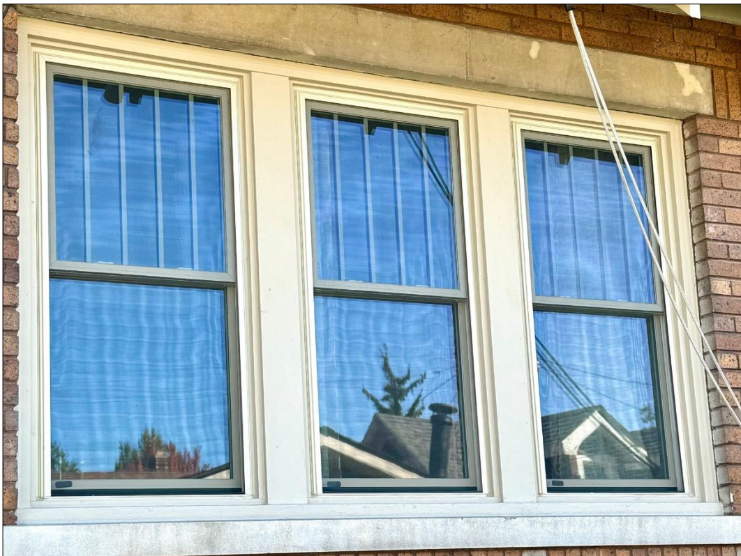
This three-unit opening is located on the rear wall. The window replacement for this opening has been completed. Staff photos, October 9, 2024.
