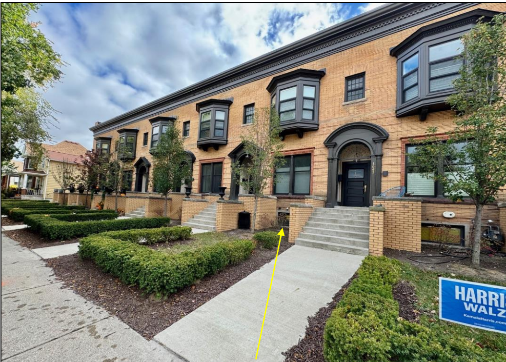
View looking southeast. Window opening that is proposed to be altered for an egress window. Staff photo, November 1, 2024.
