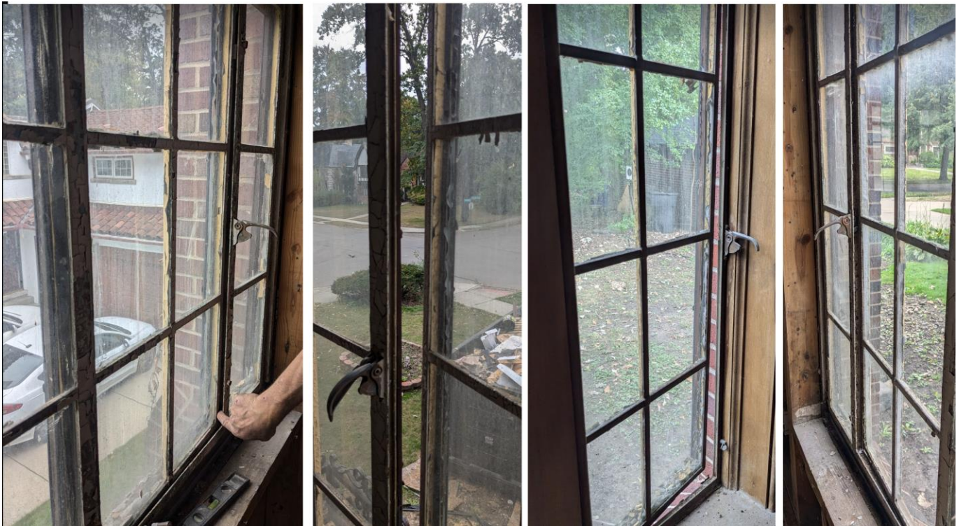
October 2024 staff photos showing warped casements.
