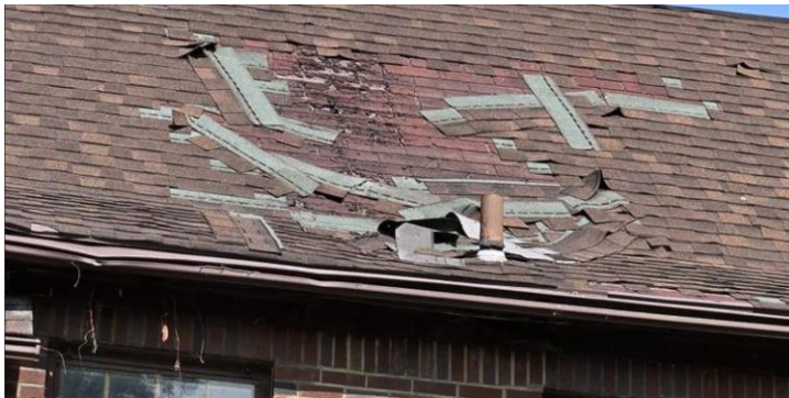
Area of prior roof deterioration. Image from August 22, 2024, application documents for roof repairs.
