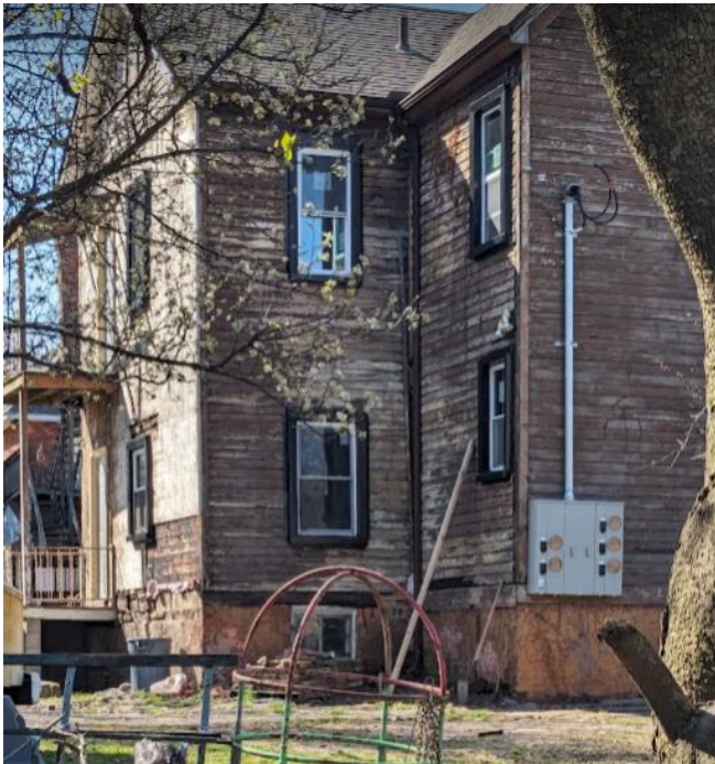
April 2024 staff photo; new electrical service connections visible at bottom right.
