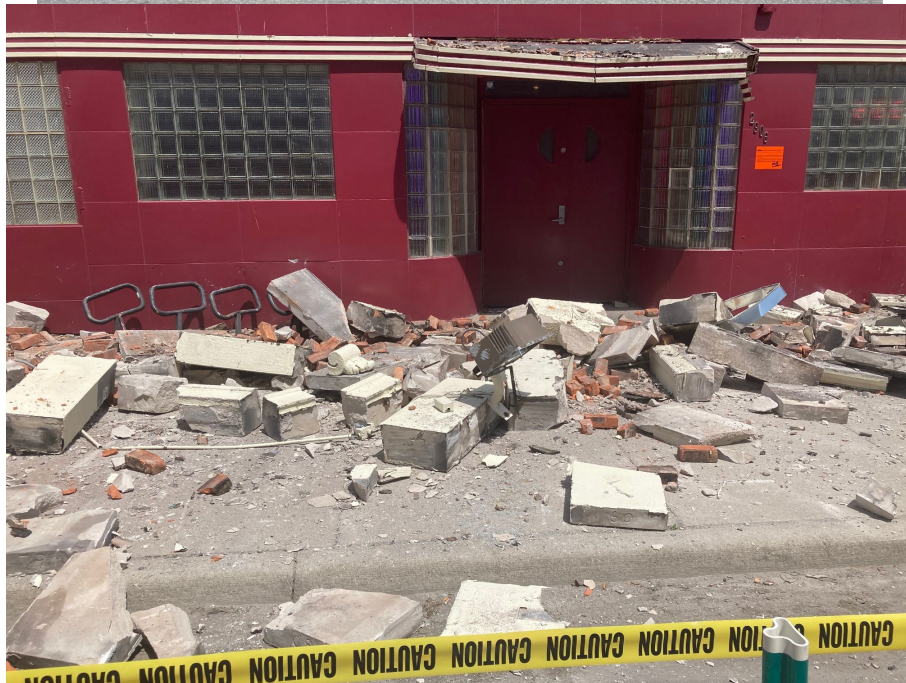
Figures 7,8: Images of the collapsed stone parapet.
