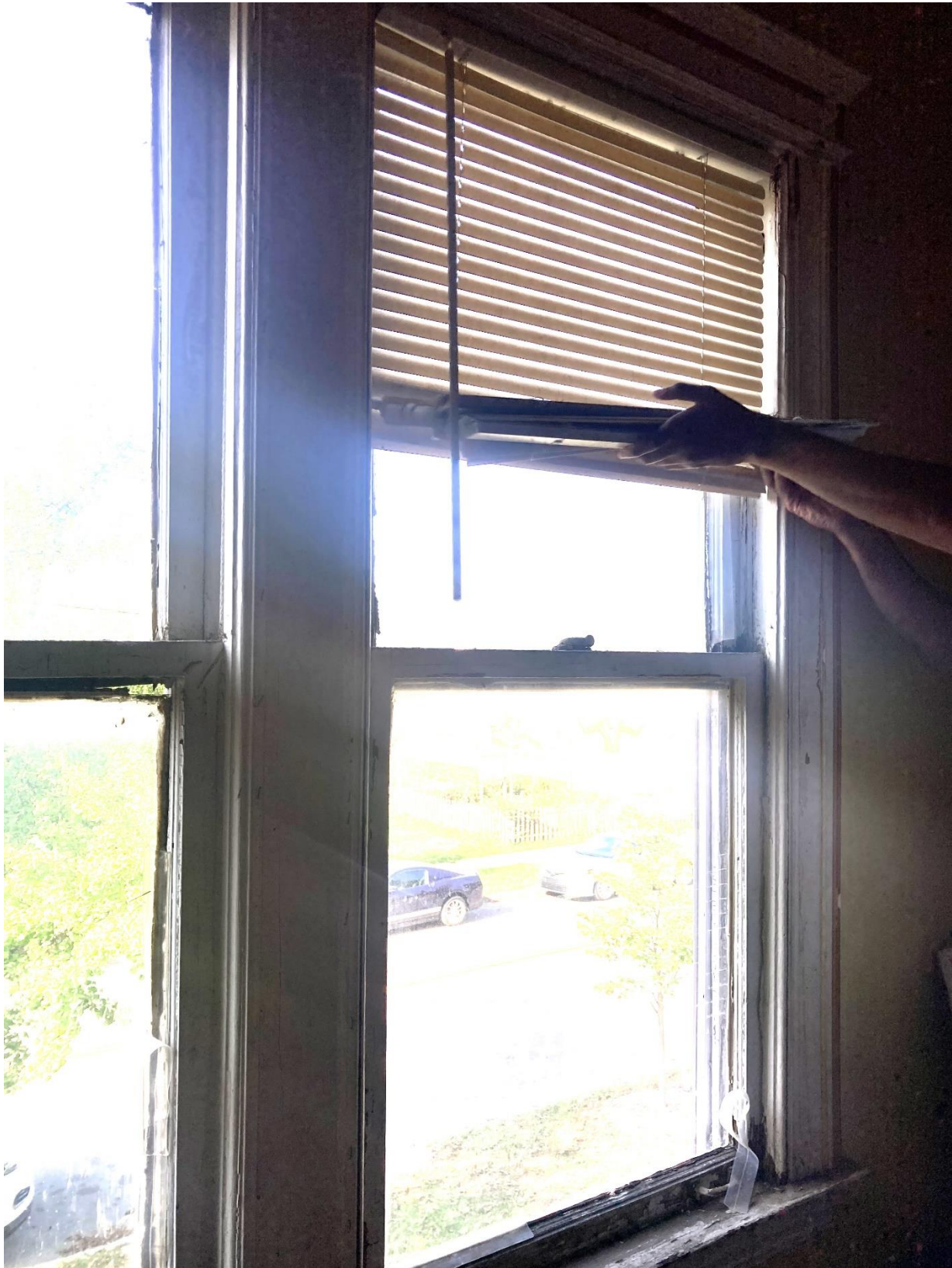
WINDOW A-02 – Gaps at sides of glass pane in both bottom and top sash; large hole at the corner of the glass pane at the bottom sash. Wood components appear to be in repairable condition. 10/3/2024 HDC staff
