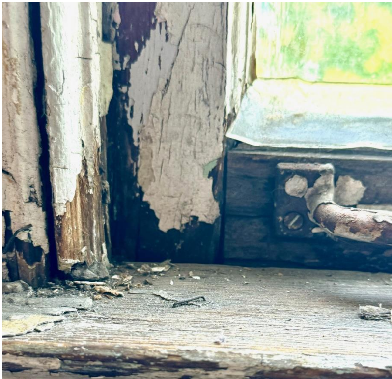
Deterioration at corner of WINDOW A-01. 10/30/2024 HDC staff
