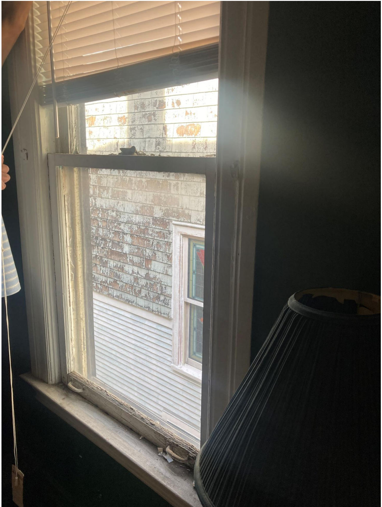
WINDOW B – Wood components in repairable condition with the exception of “spongy” bottom rail HDC staff, 10/3/2024
