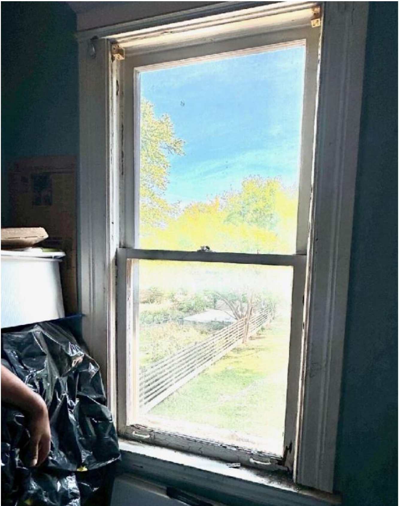
WINDOW E- Photo by HDC staff, 10/3/2024. Wood components in repairable condition with the exception of some rot at bottom rail
