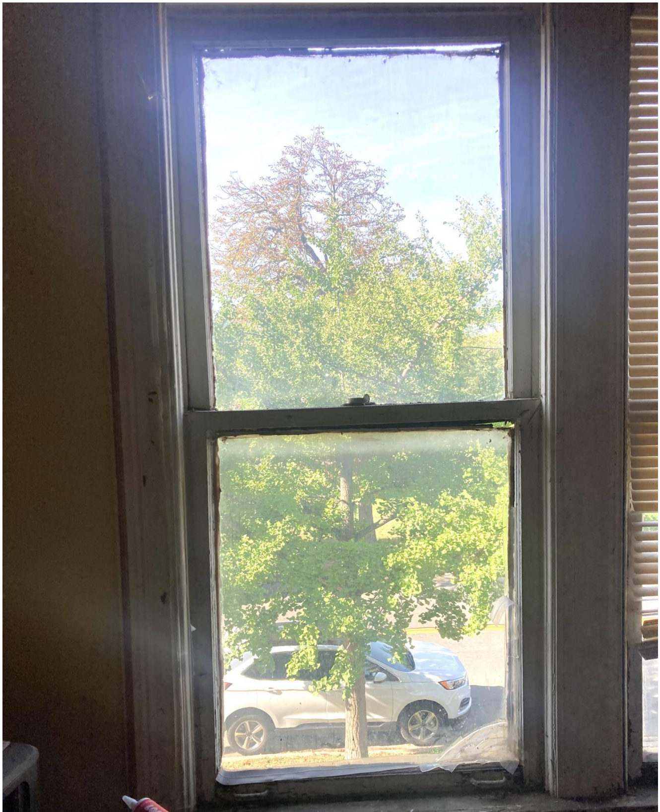
WINDOW A-01 –Gaps at top and sides glass pane in both bottom and top sash; large hole at the corner of the glass pane at the bottom sash. Wood components appear to be in repairable condition 10/3/2024 HDC staff
