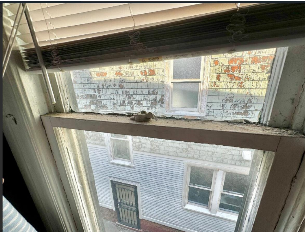
WINDOW B – Wood components in repairable condition with the exception of “spongy” bottom rail HDC staff, 10/3/2024
