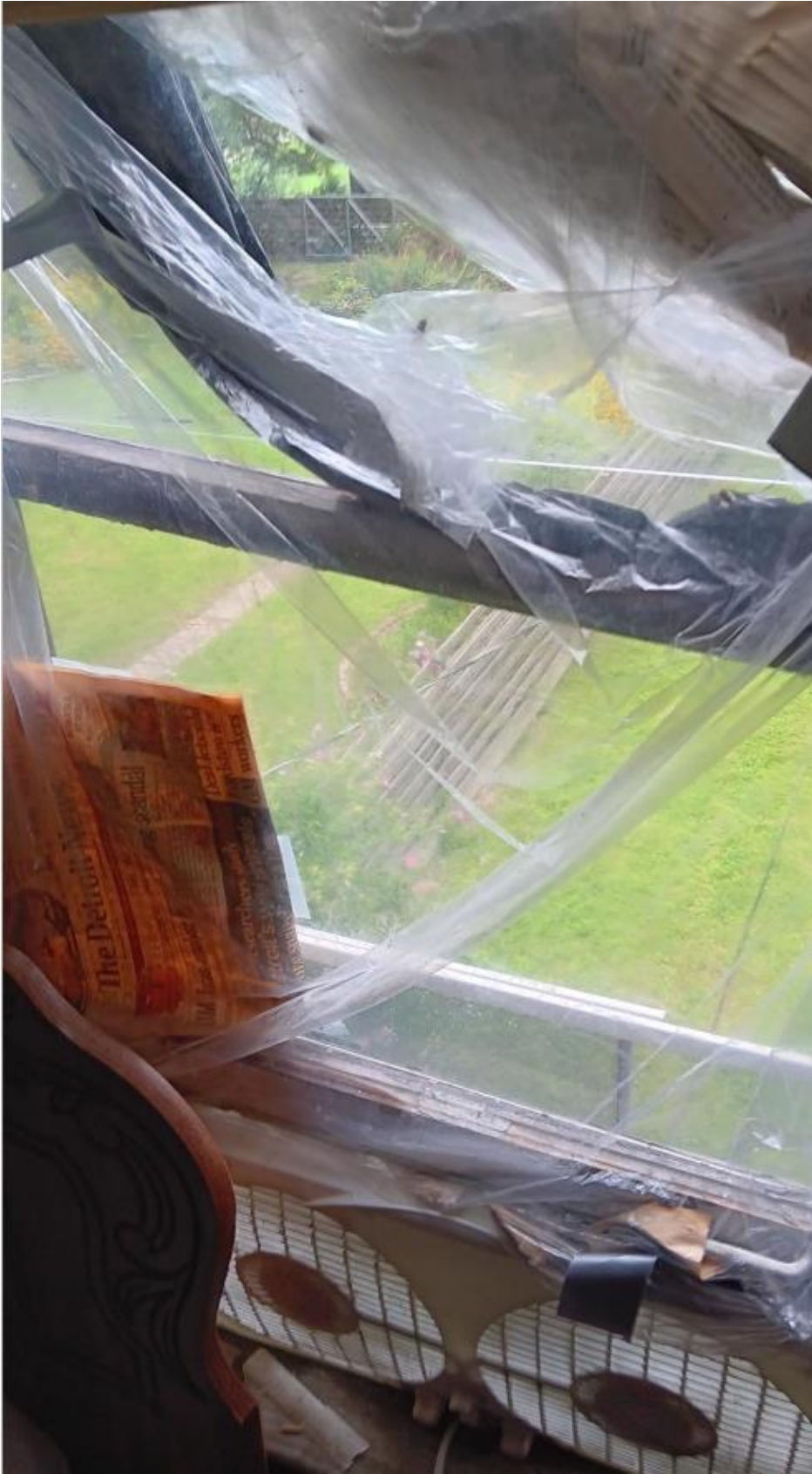
WINDOW D – Covered with plastic due to extreme air infiltration/gaps in glass panes at top and bottom sash; bottom rail at top sash is failing/about to fall off. Other wood components appear in fair/repairable condition. Photo by applicant
