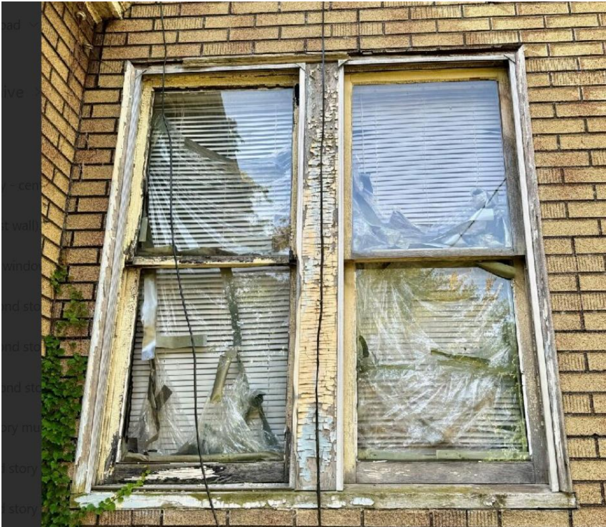
WINDOW C – No interior photos taken due to plastic covering, Staff noted that the wood components at these windows are in good condition.
