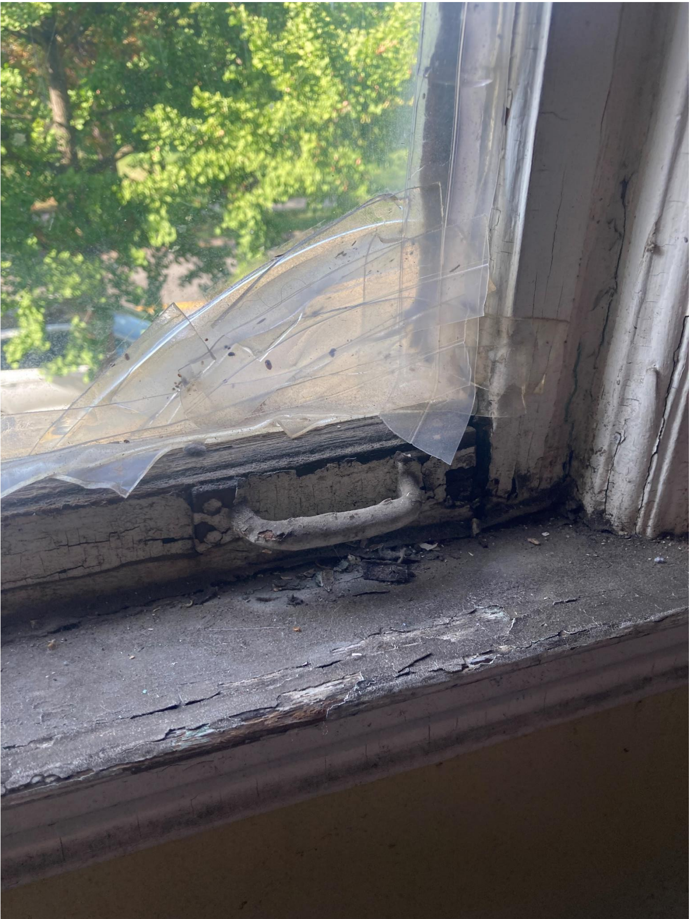
WINDOW A-01 – Large hole at the corner of the glass pane at the bottom sash. 10/3/2024 HDC staff
