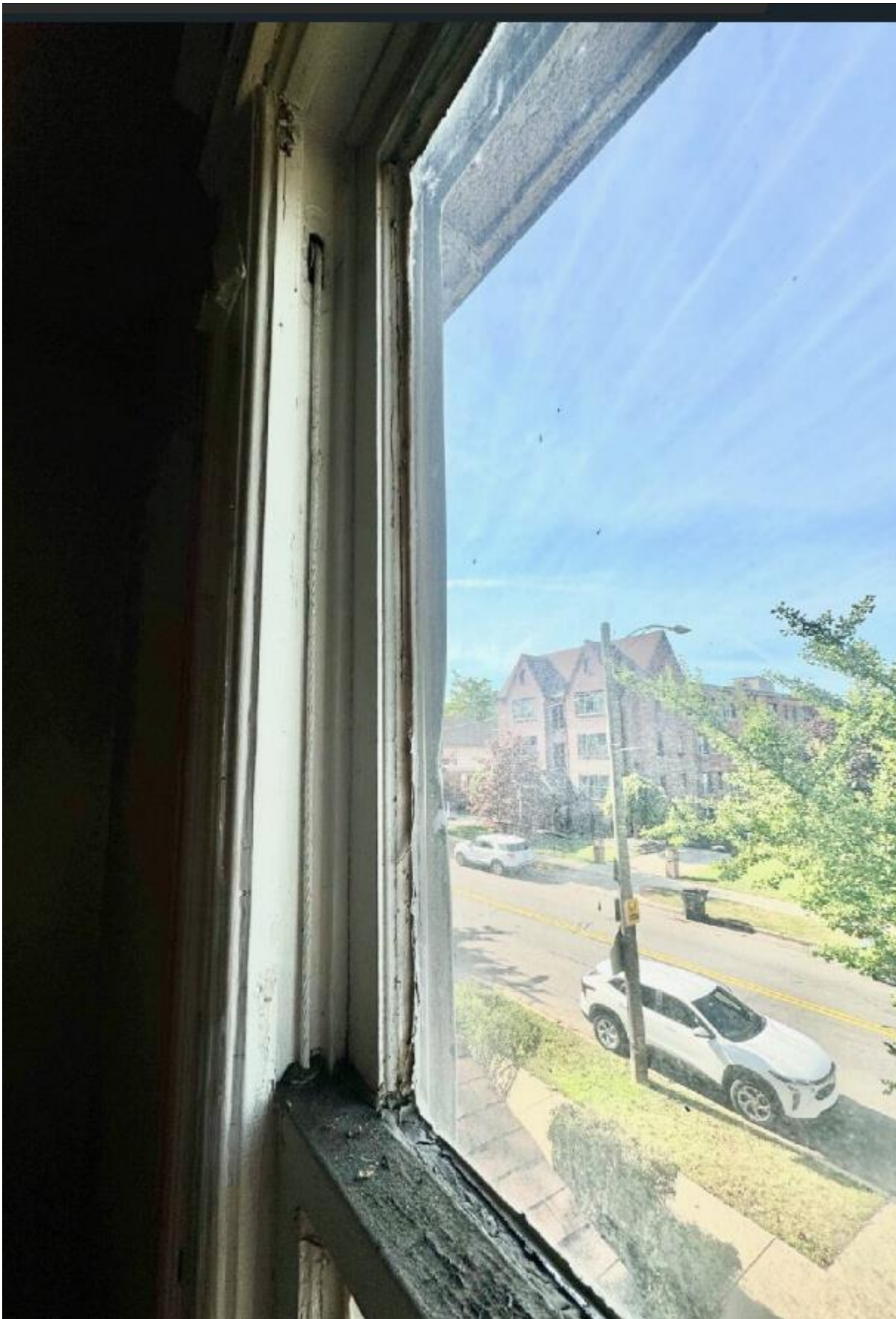
WINDOW A-01 – Showing extant sash cords. Top rail of bottom sash displays some “sponginess”. 10/3/2024 HDC staff
