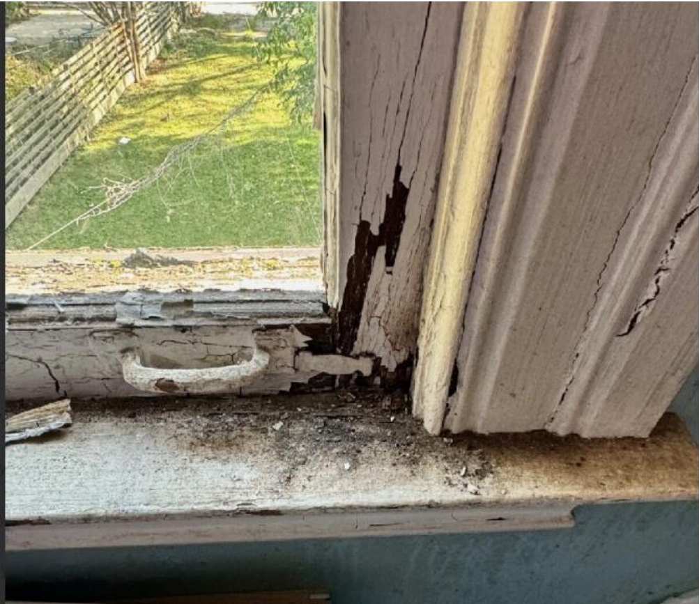
WINDOW E- Photo by HDC staff, 10/3/2024. Area of rot at bottom rail, showing previous repair
