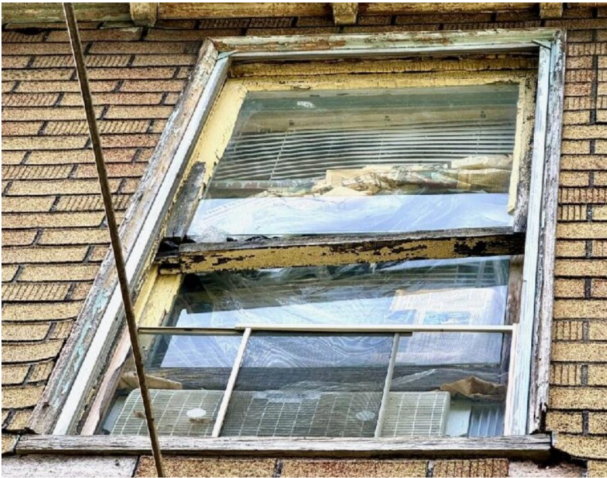
WINDOW D – Note poor/deteriorated condition of the bottom rail of the upper sash. 10/3/2024 photo by HDC staff
