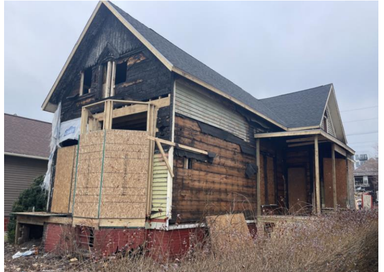
Appearance in 2/2024, after unapproved work. HDC staff
