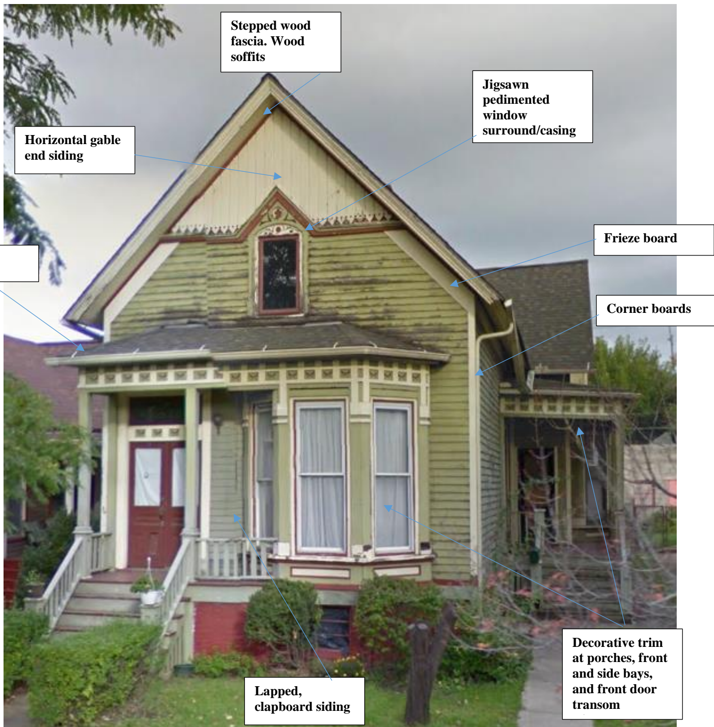
Appearance in 2016, after faux brick asphalt siding was removed. Note exposed decorative detailing at front gable end, above the front door, at the front porch roof and bay window, and at the side porch roof and bay window. Also, the front and side porch posts, piers, decking, and steps which were extant in 1983 have been replaced by this time. Source: Google Streetview
