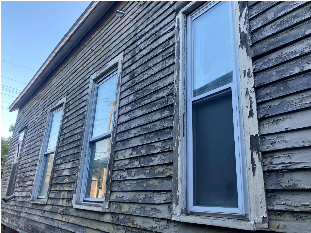
West side wall vinyl windows and remaining casing. Current condition. Photo taken by HDC staff on 9/30/2024
