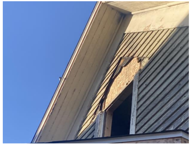
West side wall, 2 nd story gable end window. Showing current condition/missing trim. 9/30/2024 HDC staff
