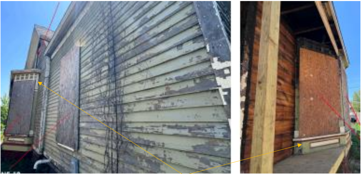
East wall bay, current conditions. Note that the historic wood detailing remains at this location despite the damage caused by the 2019 fire. Photo by applicant
