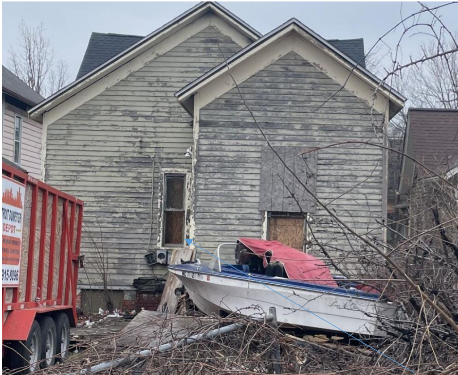
Rear, photo taken by HDC staff in 2/2024. Note that the two wood windows visible in this photo have been removed the openings covered by plywood.
