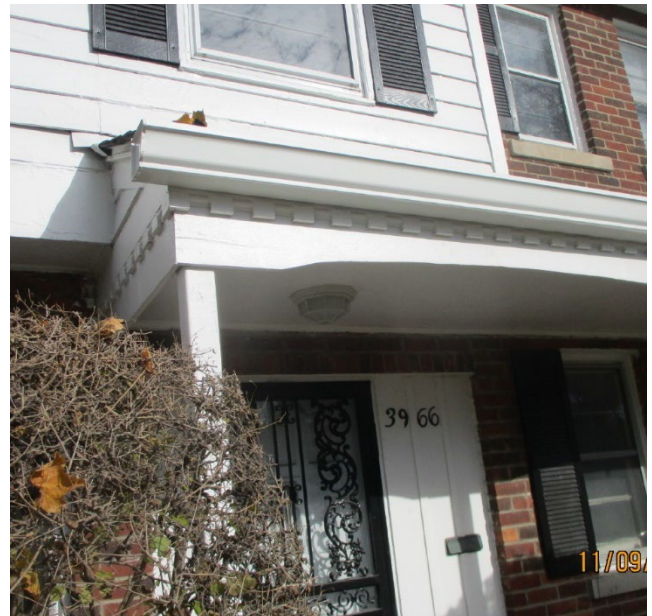
Site Photo 6, by Applicant: (South) front elevation showing detail of porch roof, front door side paneling, and second floor wood siding.
