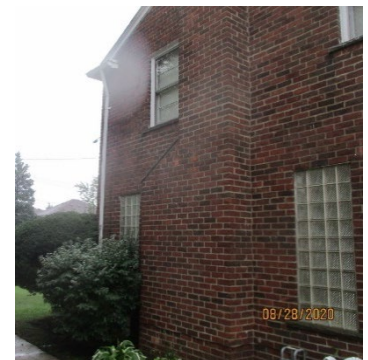
Site Photo 4, by Applicant: (East) side showing glass block windows on first floor and original windows on second floor.
