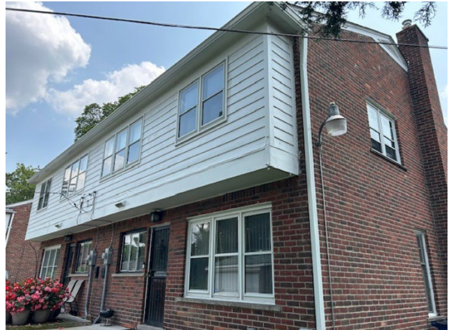
Site Photo 2, by Applicant: (North) rear side showing original double hung wood windows and doors and clap board siding.
