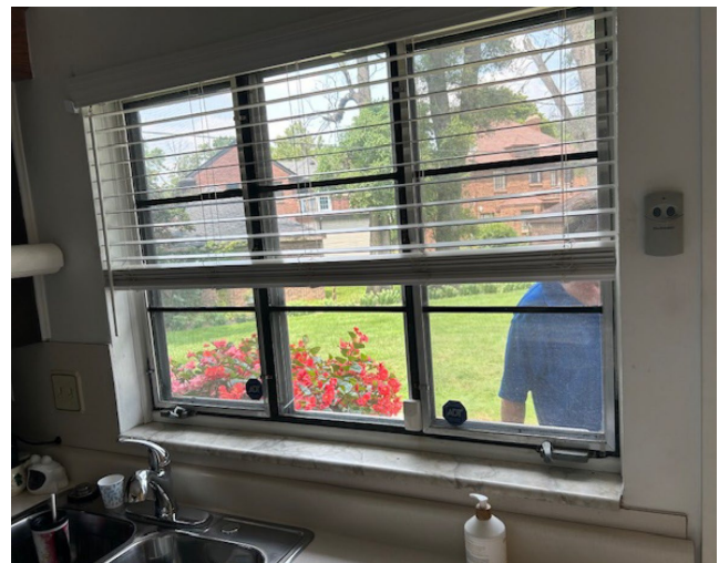
Site Photo 3, by Applicant: Interior kitchen window facing north, at (North) rear side showing casement windows with similar horizontal detailing of double-hung wood windows.
