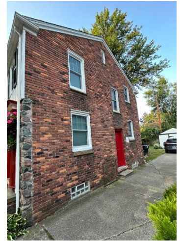
Site Photo 5, by Applicant, 2024 north (side) of the house, showing replaced windows and side door.
