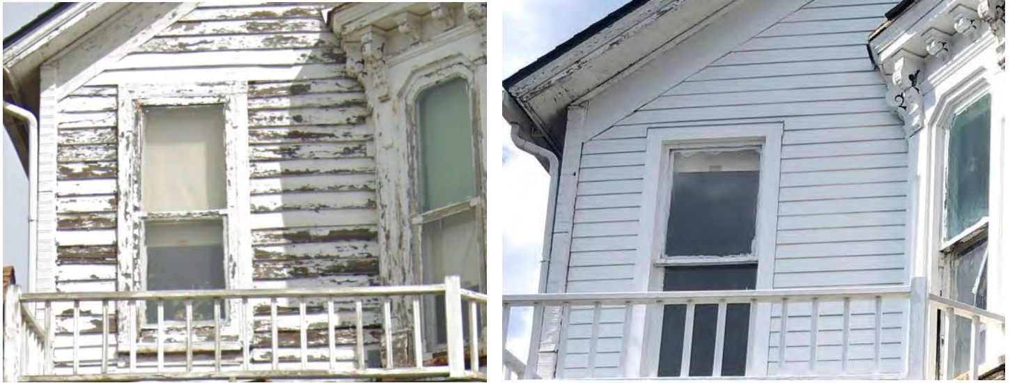
These before and after photos demonstrate changes to the historic appearance of a house by the installation of new materials. Above left: Google image, May 2019. Notice how the window casings sit in front of the wood siding. Above right: Staff photo, August 2022. It appears as though new siding was applied to this portion of the wall (between November 2020 and August 2021). The new siding is narrower in height than the old siding (there are eight clapboards spanning the upper sash in the before picture, but now there are ten). The window casing has been capped, not only losing the straightforward dimensionality of the 19 th century window casing, it also now in line with the new siding, so the dimensionality of the entire window opening has been lost.
