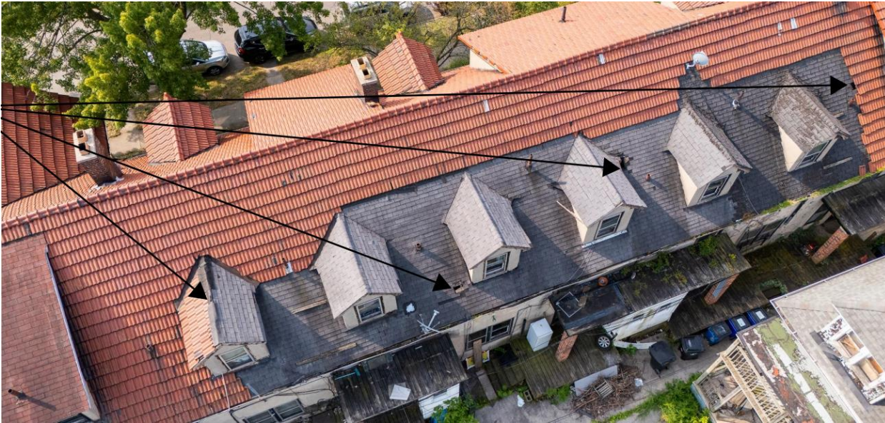
Undated photo showing rear (north) asphalt section with arrows highlighting damaged areas. Image from application materials.
