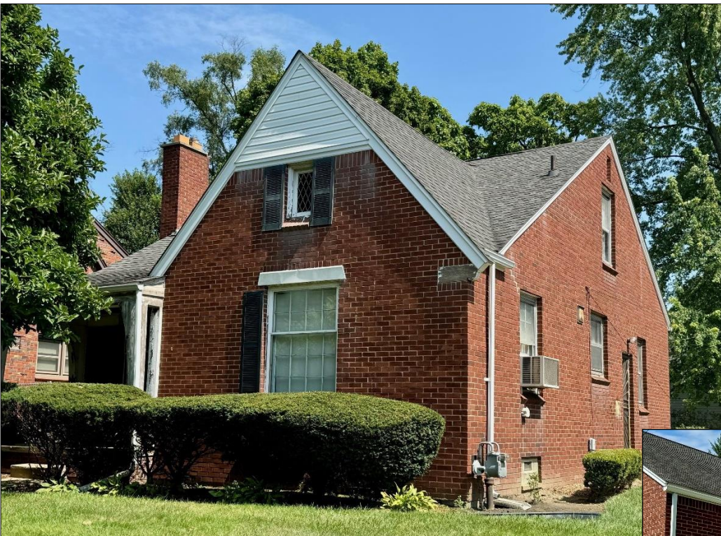
Above: Front and south side walls. A window ac unit is in the lower half of the 6-over-6 double-hung opening. Staff photo, August 27, 2024.
