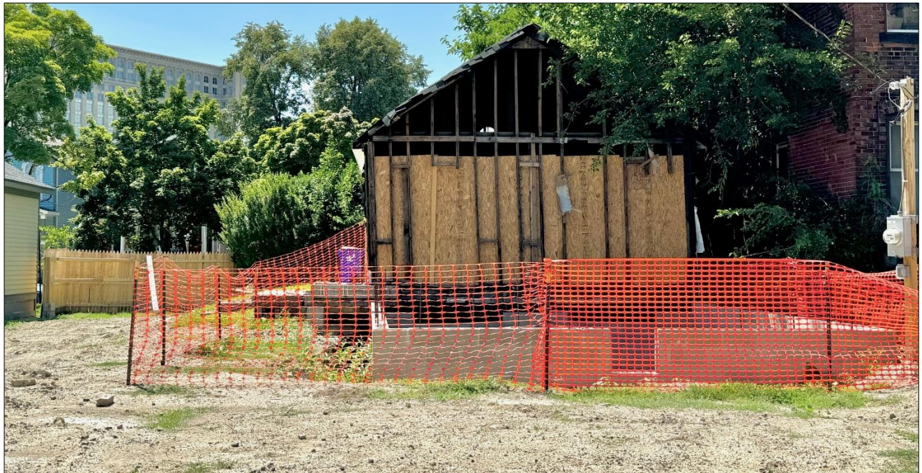
View looking west toward Wabash from alley. Staff photo, July 26, 2024. The erected concrete block foundation walls
