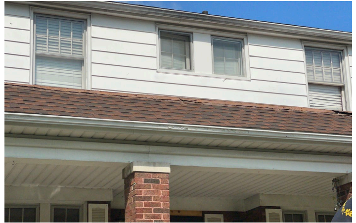
Site Photo 2, by Staff July 25, 2024: (East) front elevation showing original wood, double-hung windows with true divided light.
