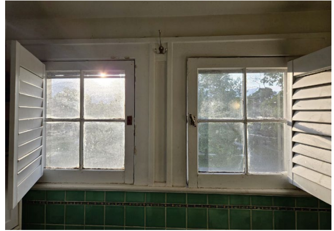
Figure 2, by Applicant: (East Interior Bathroom) Interior bathroom casement windows proposed to be replaced with vinyl windows.
