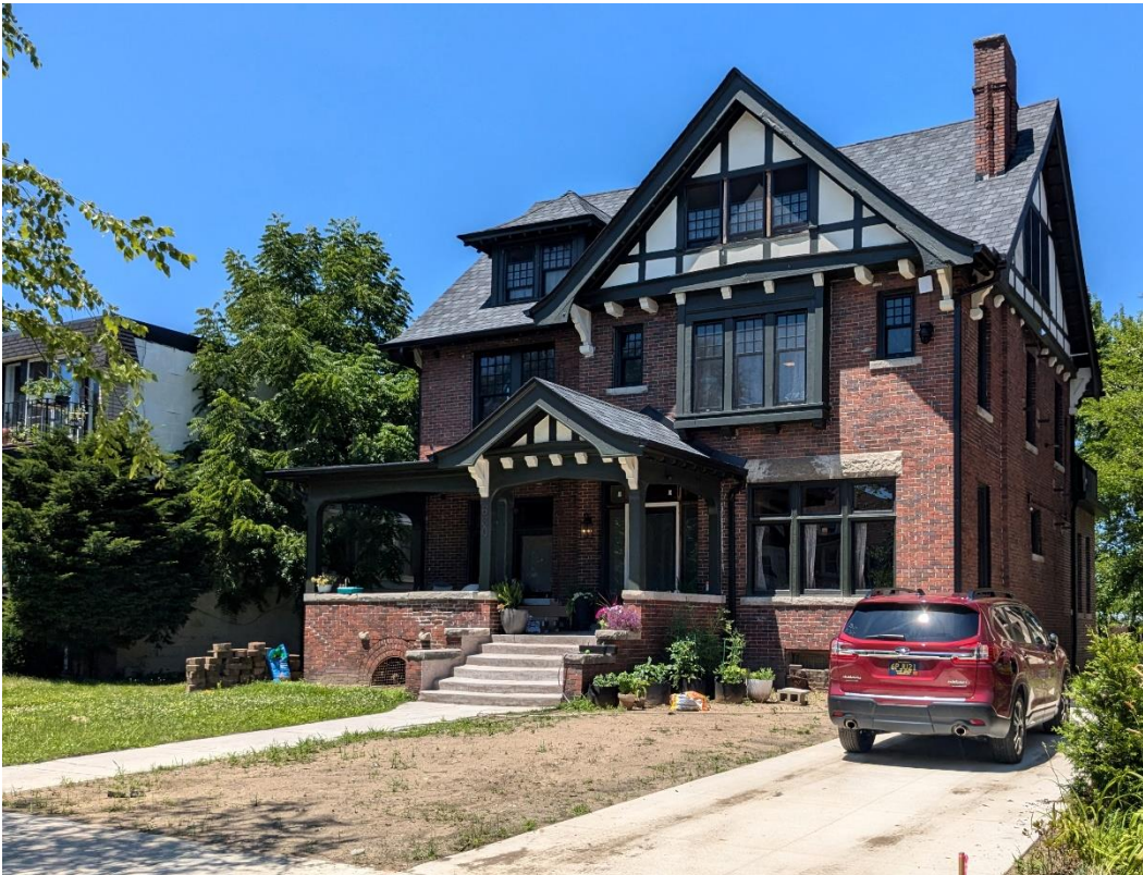
July 2024 photo by staff showing existing condition and work completed without approval.
