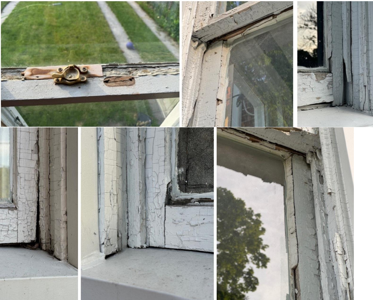
Selected images showing deterioration. Please see application documents for full, higher-resolution images.
