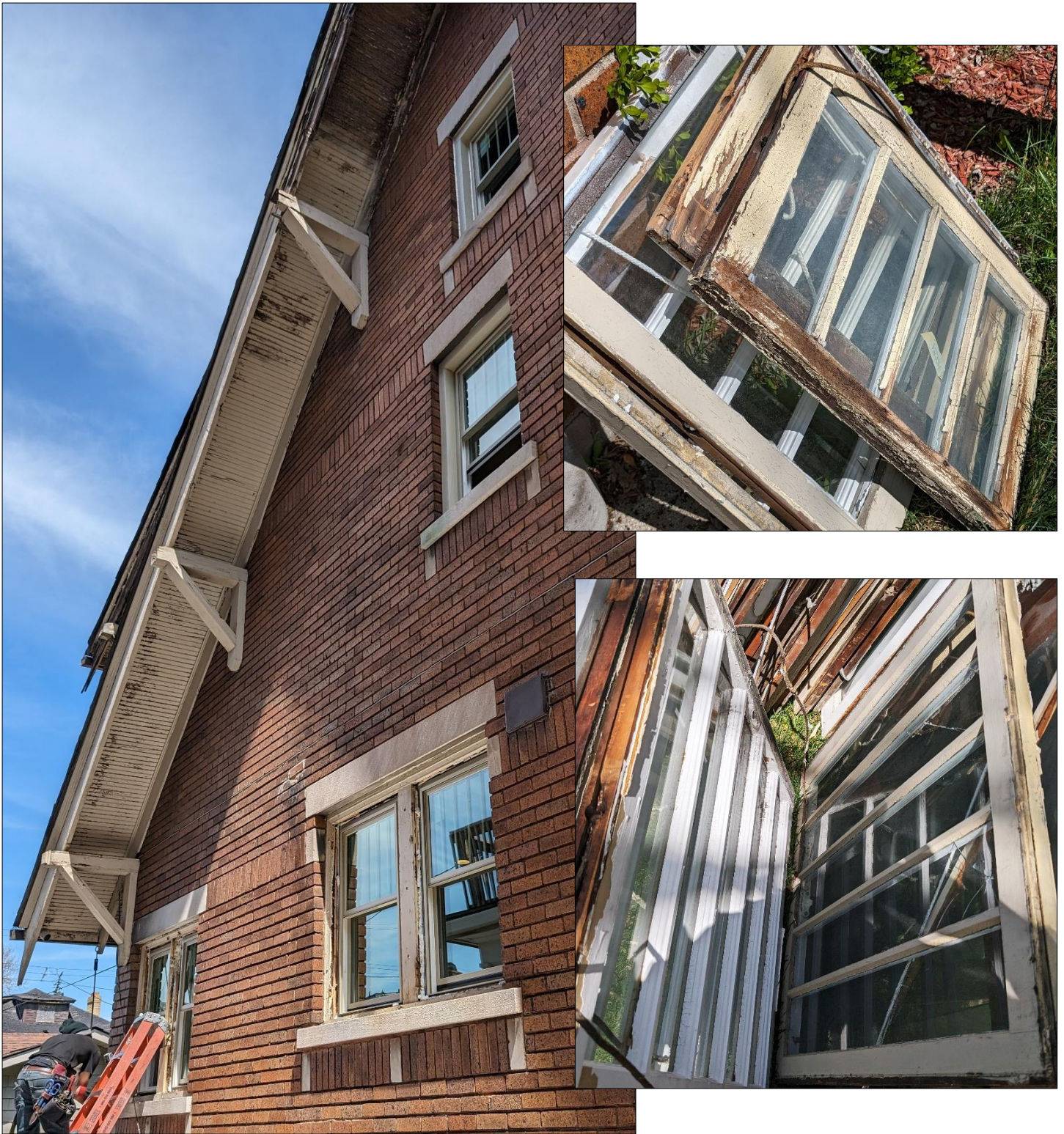
This staff photo of the west-side wall shows the reflectivity of the replacement glass, as well as the loss of dimensional profiles within the windows, due to the between-the-glass grid/muntin placement. The windows are now flat surfaces and sit in contrast with the highly detailed and dimensioned wall surfaces and applied ornament. The removed windows offer a clear comparison of the dimensional profile of true divided-light windows and a clear comparison on how these replacement windows do not match the original/historic windows.
