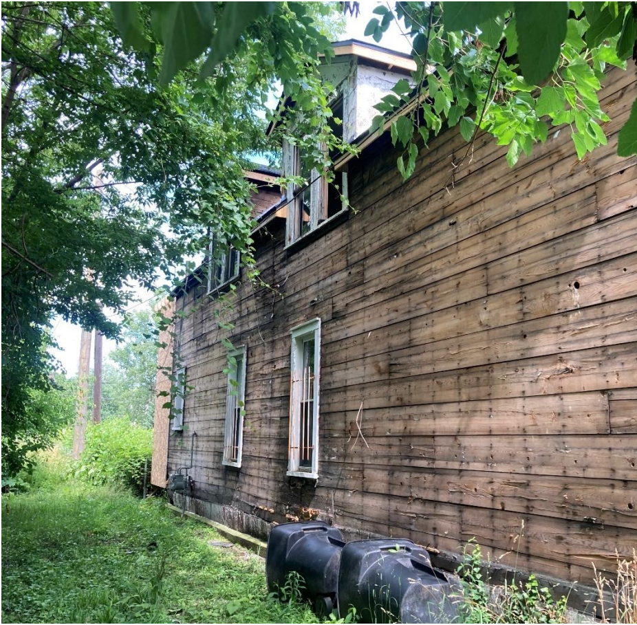
1480 Shipherd, north side. Current condition. Staff photo taken on 6/25/2024. Note that only 5 windows remain. The two windows in the western dormer and all siding and detailing/trim at the walls and roof have been removed without HDC approval
