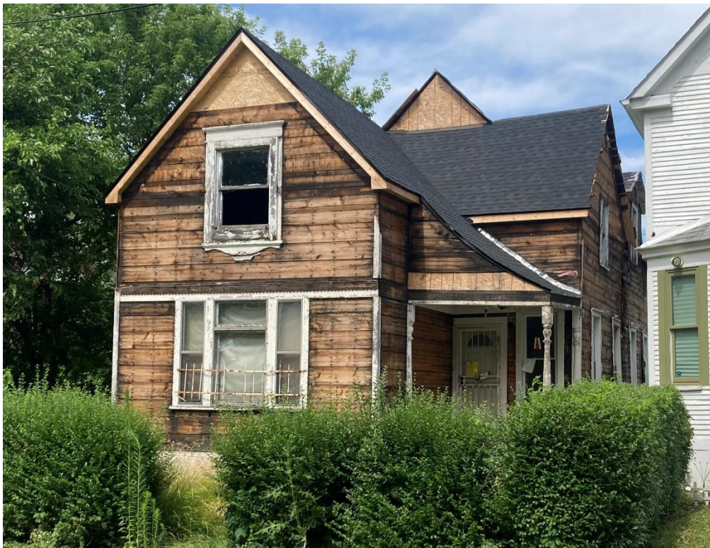
1480 Shipherd, current condition after the removal of most historic features. Compare to images on page 4. Staff photo taken on 6/25/2024
