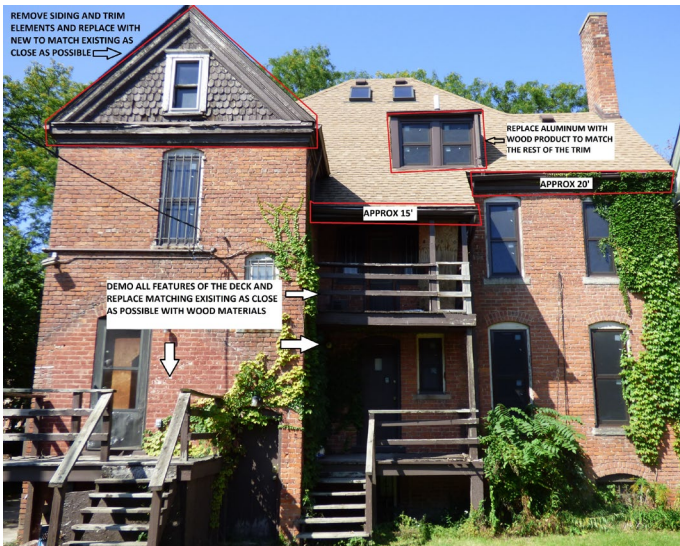
Site Photo 3, from 2020 application, date unknown: (South) rear elevation showing previous conditions of rear deck/balconies and their original footprint locations, which were approved for rebuild within these footprints. Note the scalloped siding in the gable that is reflected in the proposed stairwell enclosure.
