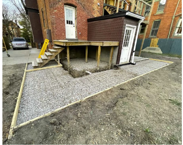
Site Photo 5, by Applicant, June 2024: (Southwest) rear elevation, showing rear stairwell enclosure, which has not yet been fully painted, and the extent of the proposed concrete paved areas.
