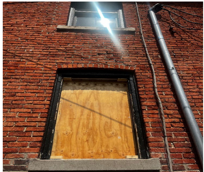
Site Photo3, by Applicant: (Looking at rear east elevation) showing location where kitchen window was removed and replaced with plywood (without approval) and showing original wood trim still in place.
