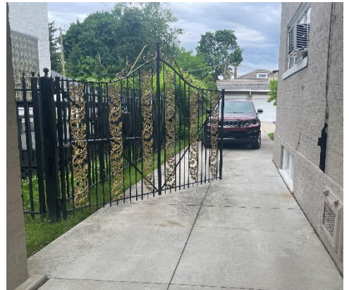
Site Photo 7 by Staff May 28, 2024: (West) side elevation, showing gate at driveway.
