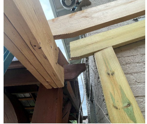
Site Photo 6 by Staff May 28, 2024: (North) rear elevation, showing elements of the arbor and gazebo construction tying the two structures together.
