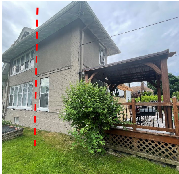
Site Photo 3, by Staff May 28, 2024: (Northeast) side and rear elevation, showing rear extension with enclosed windows at second floor. Also showing erected gazebo and deck (work completed without approval). Red dashed lines added for clarity.
