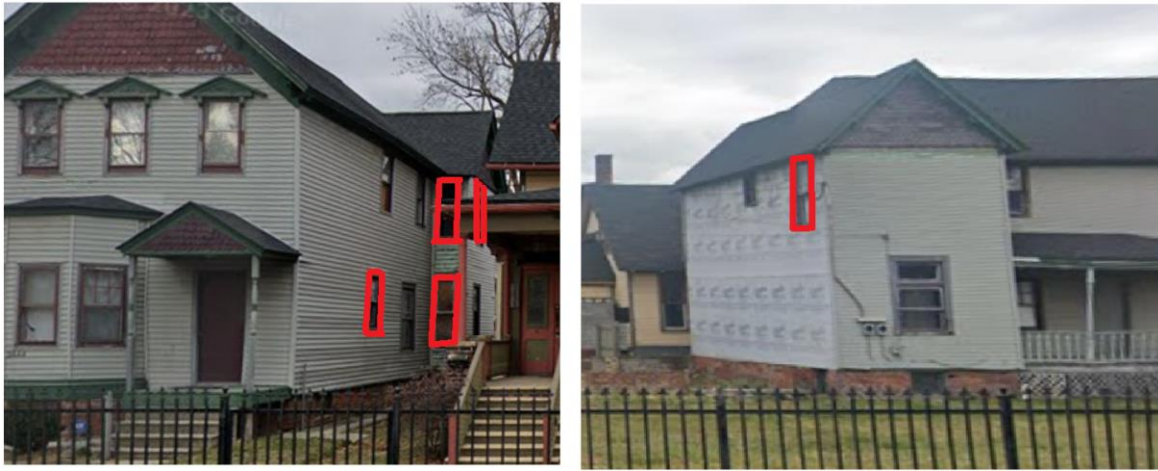
2022 Google Street View images. Red boxes added by staff to show windows that have since been removed without approval.
