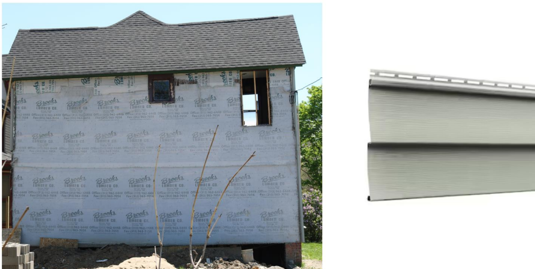
Left: Rear (north) of house where new siding is proposed. April 2024 photo by staff. Right: Proposed siding. Image from product website.
