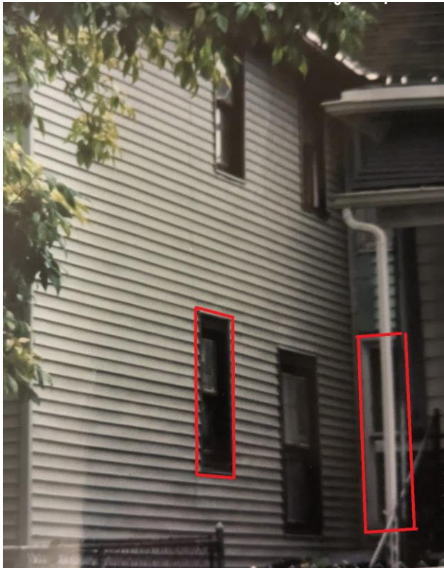
East elevation as seen in 2001 Historic District Commission staff photo, red boxes added to indicate likely historic windows that have since been removed without approval.
