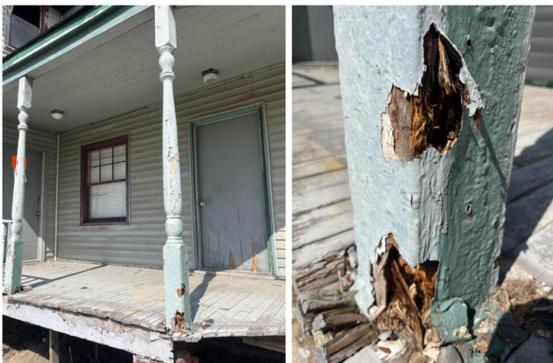
Photos of decaying porch components, from application documents.
