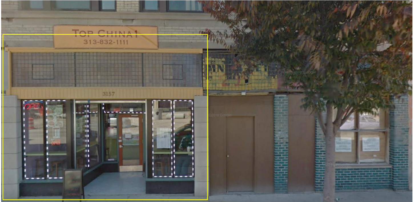
3153 Woodward. Applicant revised 2013 application in 2014 to include retain and repair of the original transom at this storefront (outlined in yellow). Google Streetview image, October 2014 to show completed project. Note that removal of red awning revealed the original transom at the storefront to the right of the targeted storefront
