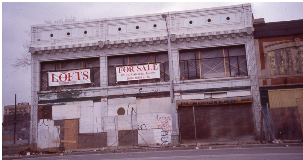
3139 Woodward, HDAB designation slide, appearance in 1984. Note that windows are in the process of being installed at the second story and first-story storefront openings are covered with plywood and an overhead door
