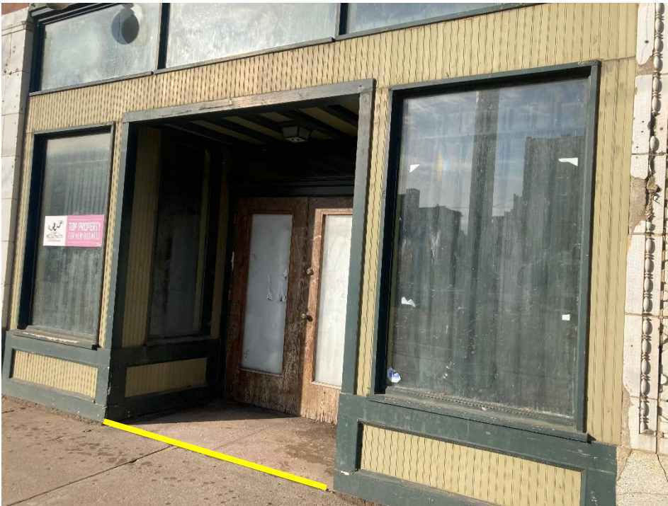
North remaining inset entrance at 3139 Woodward. Yellow line indicates where the new storefront will be located. The inset and historic terrazzo floor will be removed as the new storefront will be located flush with the sidewalk. Note that none of the actual storefront material is historic age. Only the flooring and the inset placement of the door is historic. Staff photo taken on 3/26/2024
