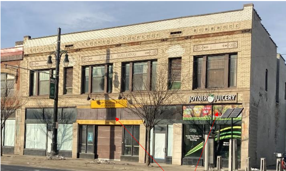
3153 Woodward, current conditions. Note that the prism glass transom only remains over the central storefront. The prism glass transom which was located above the north storefront was approved for repair in 2017. However, it was removed without approval. A salvaged prism glass transom was approved for installation at the south storefront as well. However, a new aluminum transom was installed without approval. Staff photo taken on 3/26/2024, facing southwest
