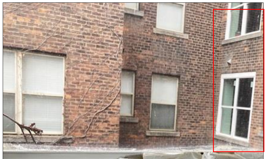
Applicant photo. Recently installed non-approved vinyl windows are in the red lined box.
