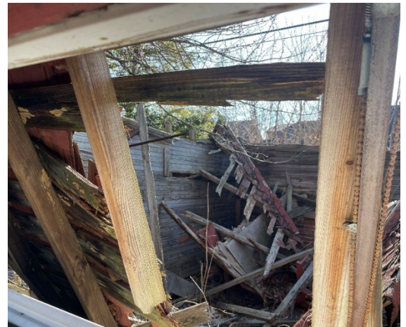
Site photo 4, by Staff February 23, 2024: (facing south) interior of garage showing collapsed roof.
