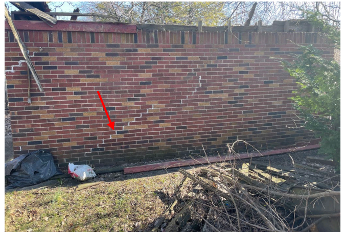
Site Photo 3, by Staff February 23, 2024: (facing east) west wall of garage, showing brick displacement and cracking along the wall.
