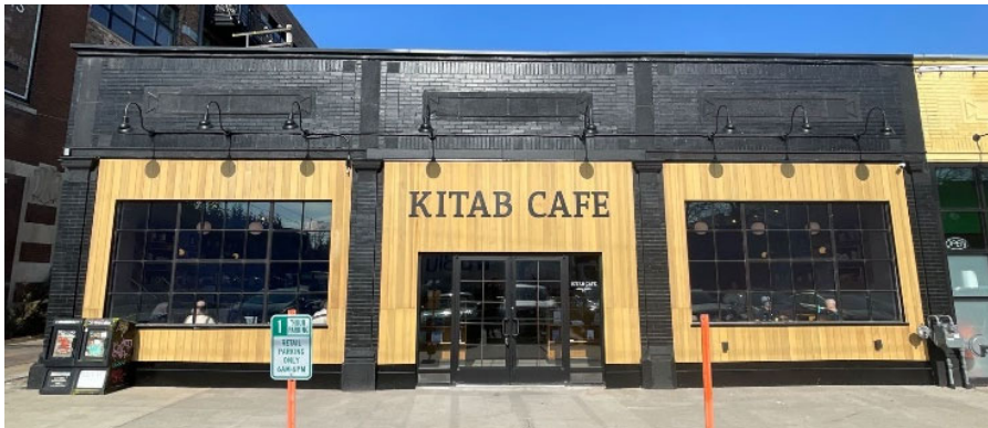
Site Photo 5, by Staff February 23, 2024: (North) front elevation, showing current, unapproved paint and sign installation conditions.
