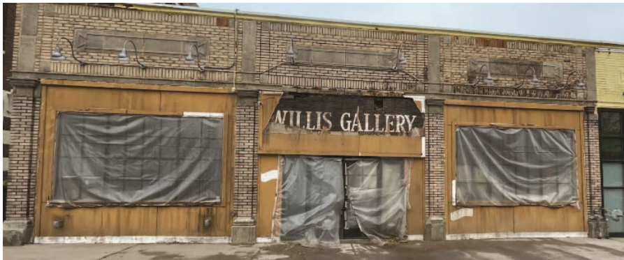
Site Photo 4, by Applicant December: (North) front elevation, showing approved paint removed conditions.
