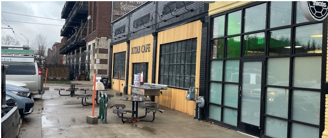
Site Photo1, by Staff January 11, 2024: (North) front elevation, showing current, unapproved paint and sign installation condition.
