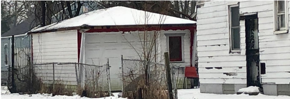
19337 Lyndon – 1963/12/63 - Garage // Dwelling – 1941/07/01 -no garage was shown on 1950 Sanborn map, so this is likely the first garage on this property.
