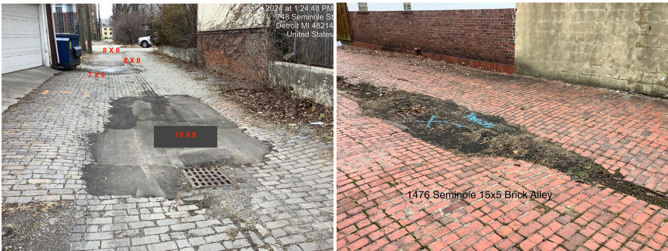
Figure 4: Examples of typical repair locations provided by the applicant.
