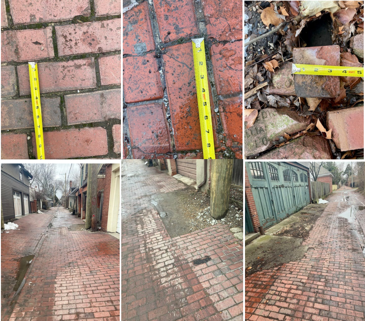
Figure 6: Images showing the dimensions and conditions of the paving in the alleys north of Lafayette.
