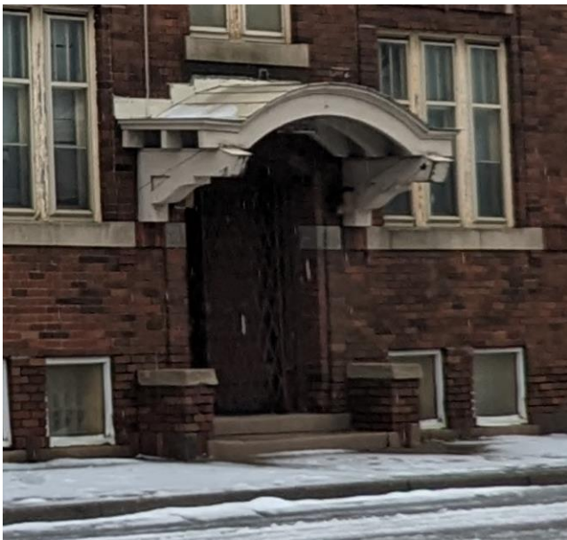
North-facing canopy (located on original, 1912 building) proposed for removal. No replacement is proposed. January 2024 photo
