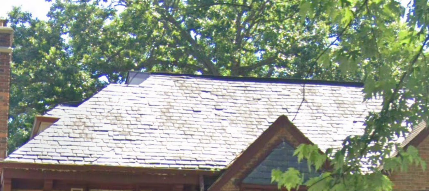
Figure 5: Image of 19650 Canterbury from 2022 showing deterioration of the slate roof. Google Street View
