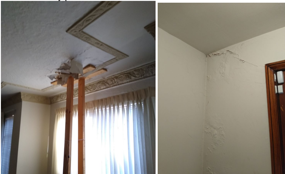
Figures 3,4: Images provided by the applicant showing paint and plaster damage at the second floor of the home.
