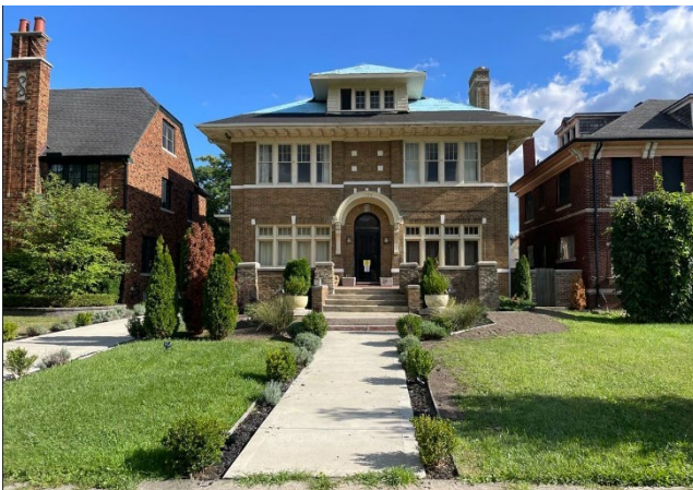
Site Photo 1, by Staff August 25, 2022: (Northwest) front elevation, showing removed clay tile roof and partial asphalt roof installation.
