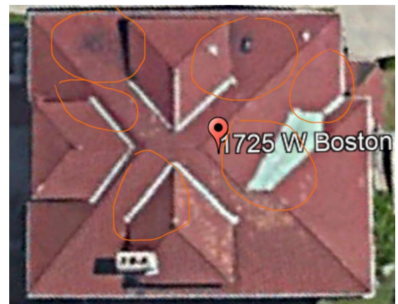
Aerial 2, by Applicant, indicating locations of leaking areas of the house's roof (red).
