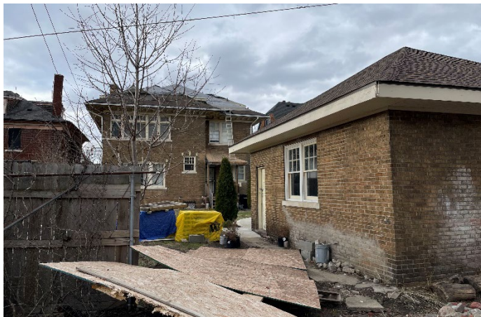
Site Photo 3, by Staff March 25, 2022: (Southeast) rear elevation and garage, showing partial installation of new asphalt roof.
