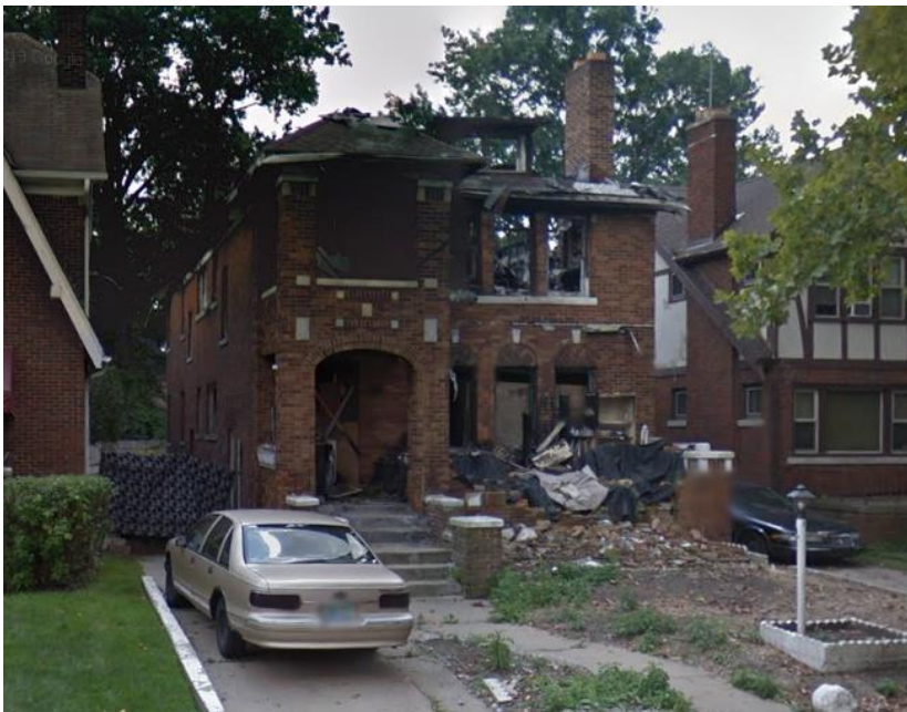
Damaged house at 4305 Buena Vista. 2013 Google Maps photo.
