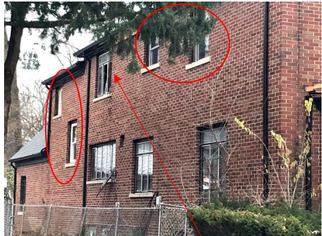
Staff photo, November 2023. The damaged casement, shown on the previous page, is visible here. Installed vinyl windows are circled.
