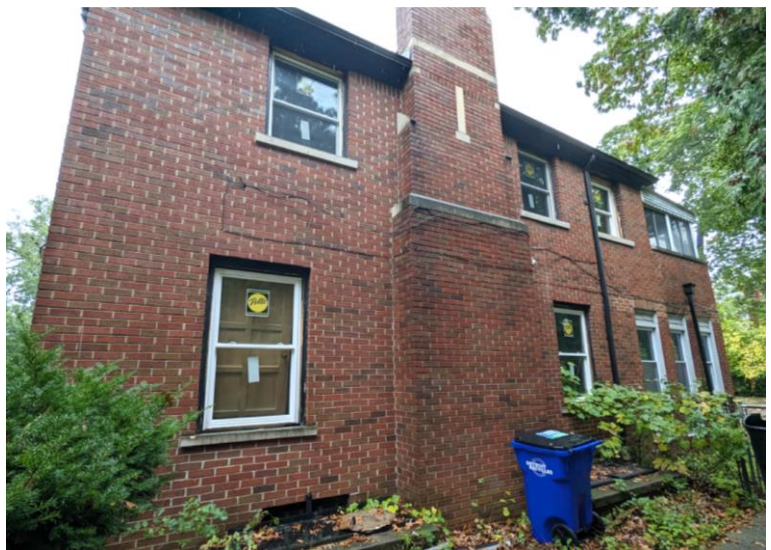
Applicant photo. All the historic window sash on this elevation have been replaced with vinyl windows.
