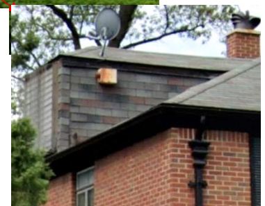
Right: Google street view, May 2019. This partial close-up view shows the previous condition of the dormer. It had been covered with asphalt shingles prior to the district’s designation.
