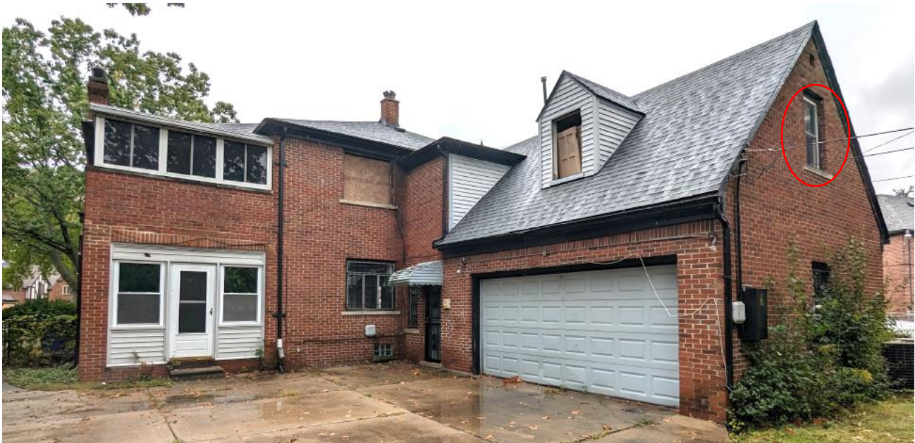
Applicant photo. At the second floor of the garage, one vinyl window has been installed, and two openings (one at garage, and one at house) have had window sash removed. Historic sash remains at the first floor of the house and garage.
