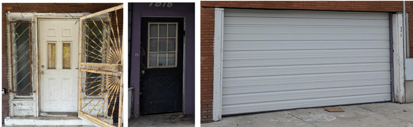
Non-historic doors to be replaced. Leftmost image from application materials, other images from December 2023 staff site visit.
