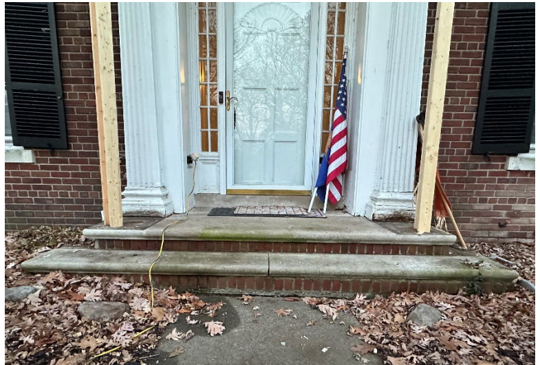
Site Photo 4, by Applicant: (East) front porch existing conditions, showing the original dimensions of the threshold, upper landing, and the lower step.
