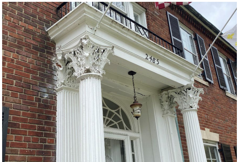
Site Photo 5, by Applicant: (East) front porch existing conditions, showing the original capitals and water damage over the doorway.
