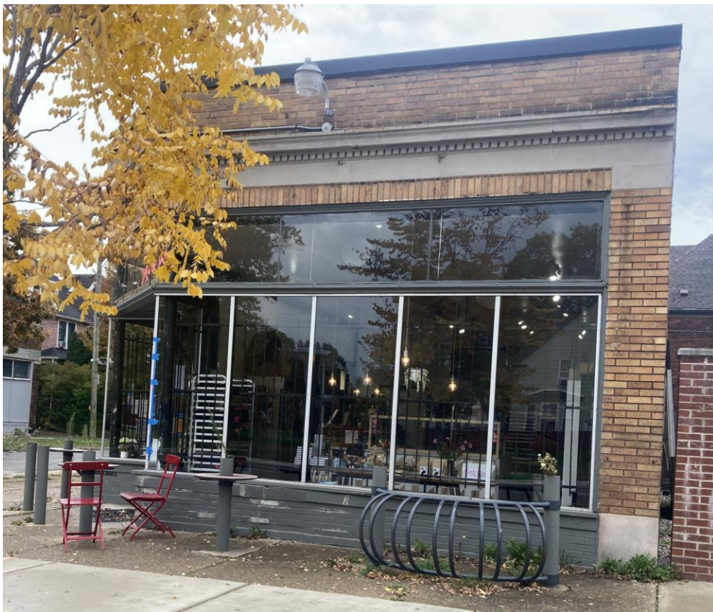
Primary storefront proposed for replacement with new aluminum storefront. Wood doors, aluminum windows, wood trim, wood transom, and penny tile will be removed.
