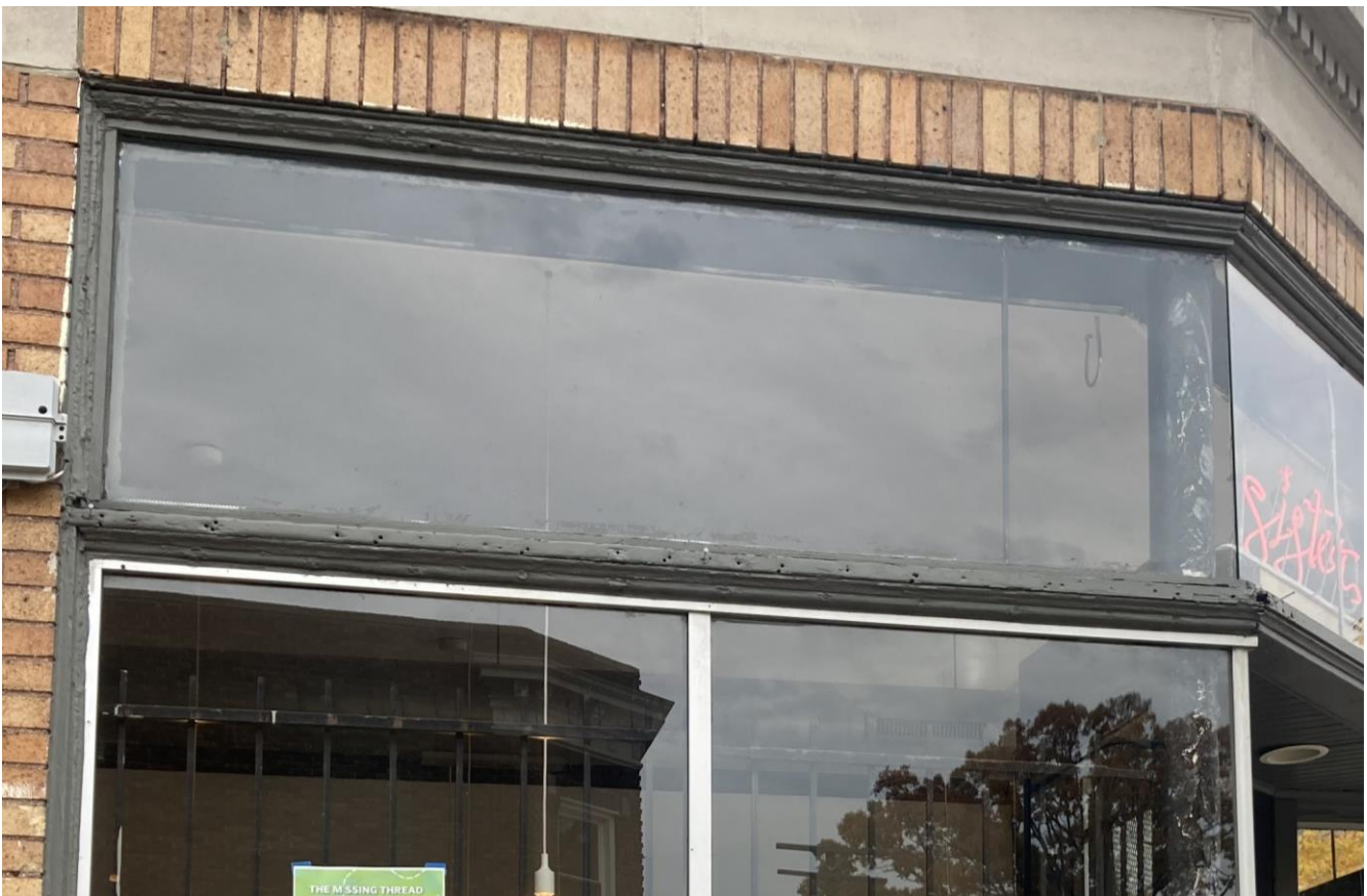
Transom at main entrance/primary storefront., facing west. Note trim profile. Staff photo taken 10/28/2023
